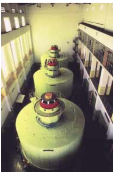
Turbines turn generators at a hydroelectric power plant. (Luis Casaneda/The Image Bank)
