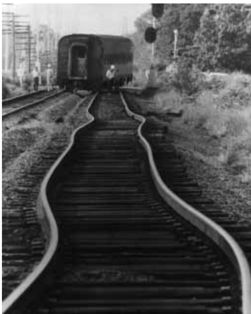
Thermal expansion: The extreme temperature of a July day in Asbury Park, NJ, caused these railroad tracks to buckle and derail the train in the distance. (AP/Wide World Photos)
