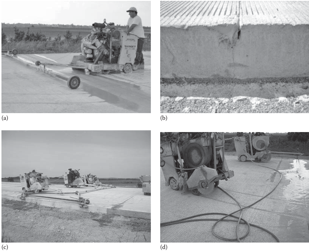
FIGURE 17.16 (a–d) Joint sawing operations in PCC pavements. (Courtesy of Wouter Gulden, ACPA-SE Chapter, Duluth, GA.)
