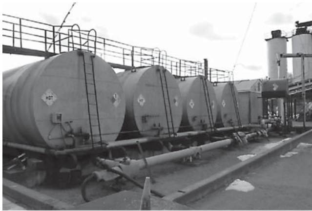
FIGURE 16.10 Asphalt storage tanks. (Courtesy of Matthew Teto, All States Asphalt, Sunderland, MA.)
