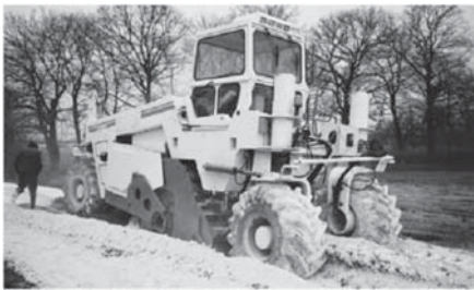
Lime stabilization with Wirtgen WR 2500 Working width: 8 ft, Working depth: 0–20 in. Engine output: 690 HP, Weight: 63,000 lb
