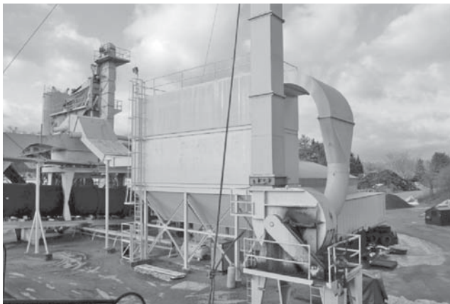
FIGURE 16.9 Baghouse. (Courtesy of Matthew Teto, All States Asphalt, Sunderland, MA.)
