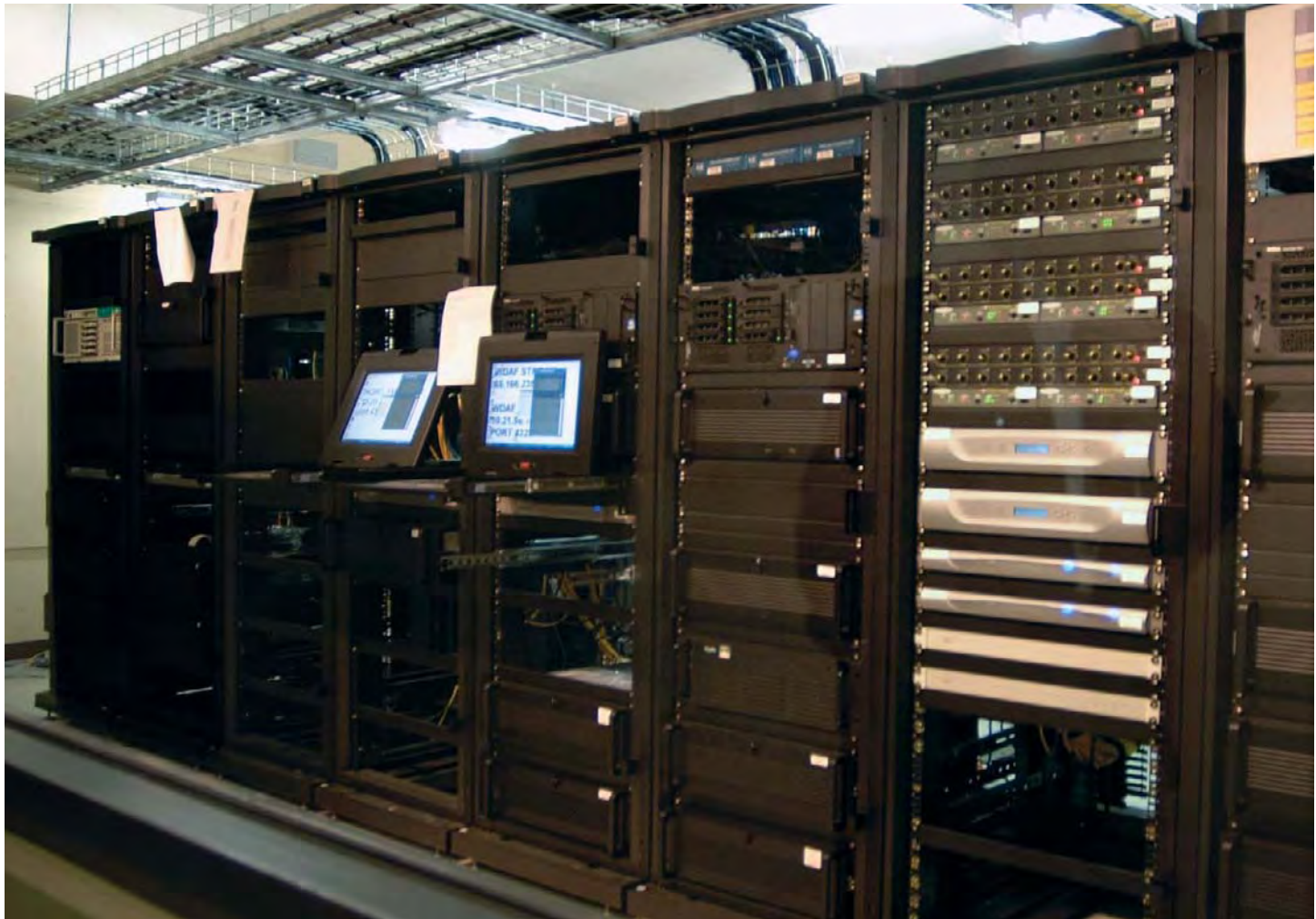
Engineering TOC Entercom Communications Kansas City
