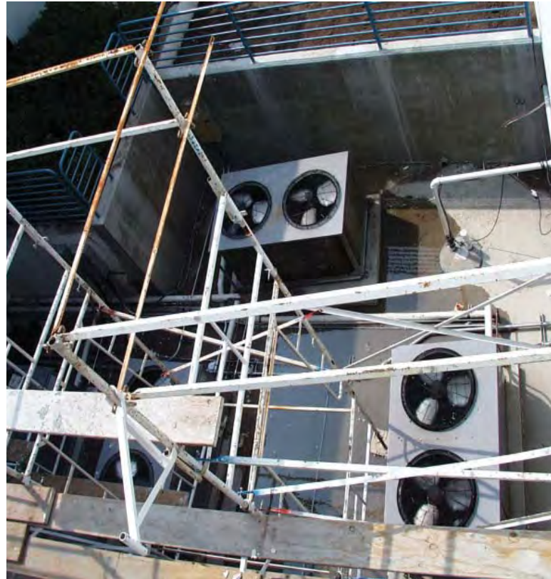
Roof Top Mechanical Equipment
