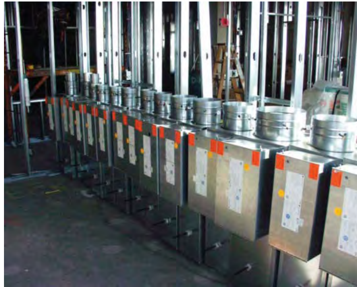
Mechanical VAV Boxes
