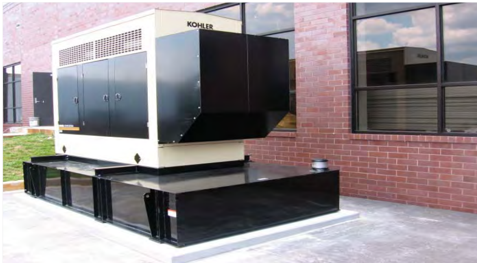
Back Up Generator CBS Radio Baltimore
