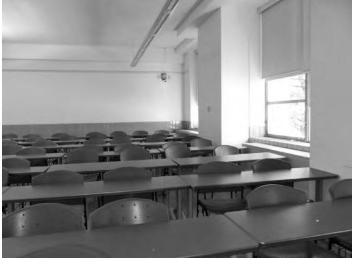
Figure 6–10 Displacement induction units in classroom building. Asif Syed
