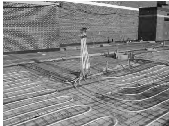
Figure 2–5b Radiant pipe manifold. Photo taken and provided by BHC Architects
