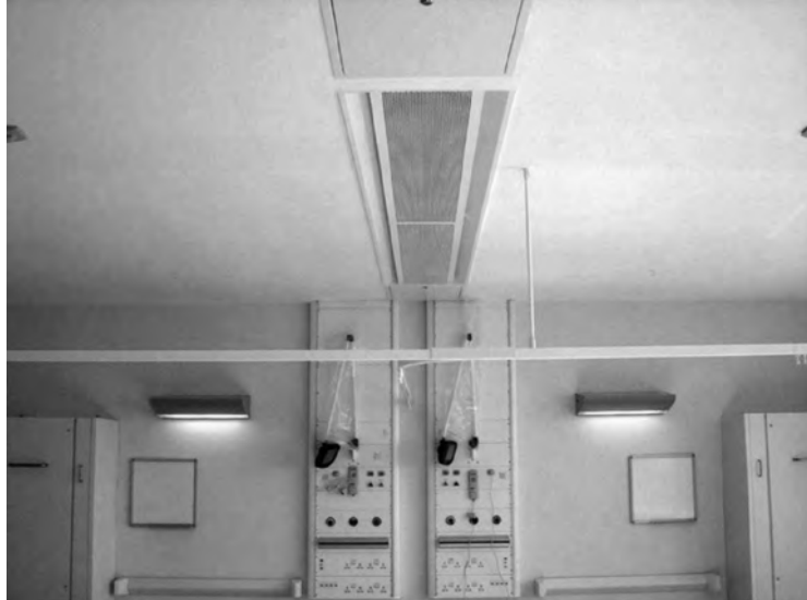
Figure 4–10 Chilled beam use in a hospital. TROX Technik
