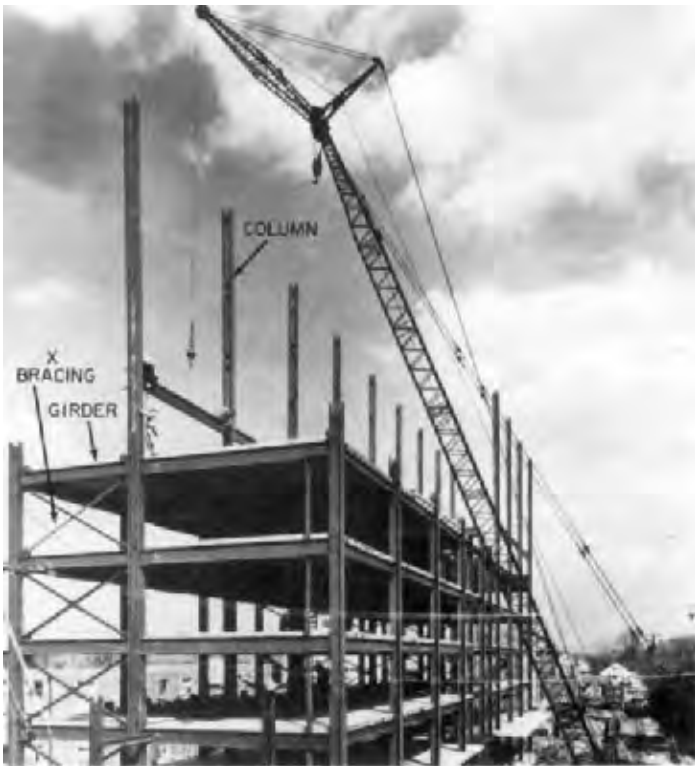
FIGURE 1.3 Structural-steel skeleton framing for a multistory building. (Courtesy of the American Institute of Steel Construction.)
