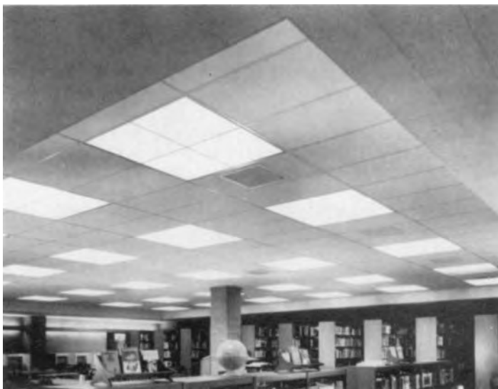
FIGURE 11.98 Library ceiling comprising both acoustical panels and acoustical tiles, integrated with lighting panels. ( U.S. Gypsum Company. )
