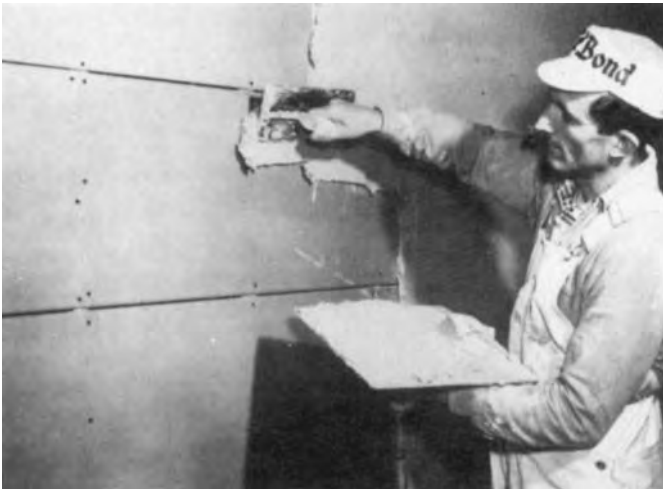
FIGURE 11.22 Application of a base coat of plaster to gypsum lath. (Gold Bond Building Products, a National Gypsum Division.)
