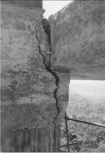
Figure 1.2 Edge beam starting to separate from column.
