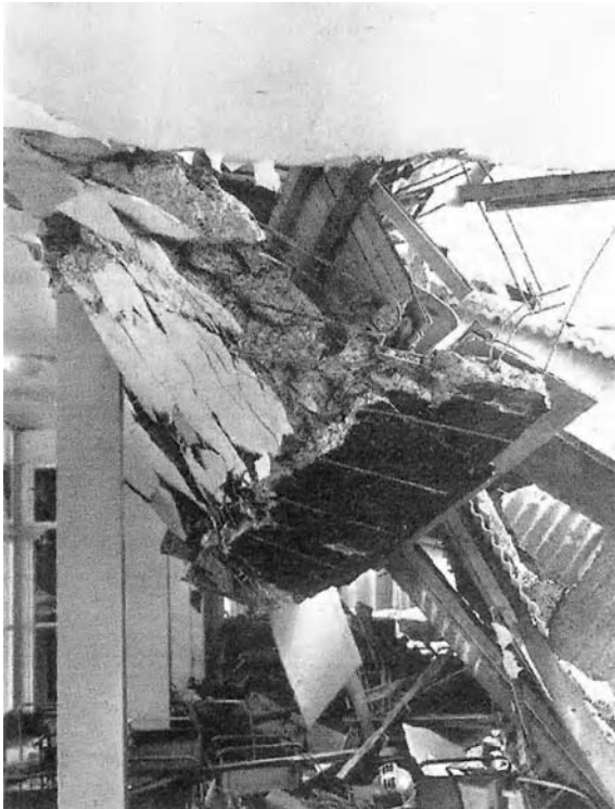
Figure 6.6 Part of roof that collapsed on chairs below. (From Scott, G.A., Building Disasters and Failures , Construction Press Ltd., Lancaster, 1976. With permission.)
