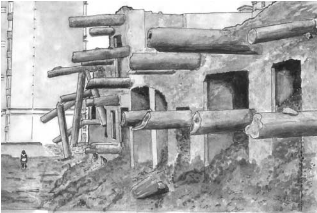
Figure 10.8 View of piles that failed in shear. (Courtesy of Gillian Whittle; redrawn from Reuters, http://www.telegraph.co.uk/news/worldnews/asia/china/5685963/Nine-held-over-Shanghai-building-collapse.html .)
