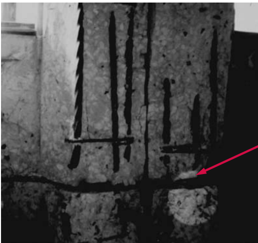
Figure 8.17 Spalling of mullions. (Courtesy of Poul Beckmann.)
