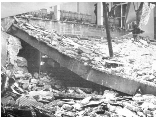
Figure 6.7 Collapsed roof lying on floor below. (From Scott, G.A., Building Disasters and Failures , Construction Press Ltd., Lancaster, 1976. With permission.)
