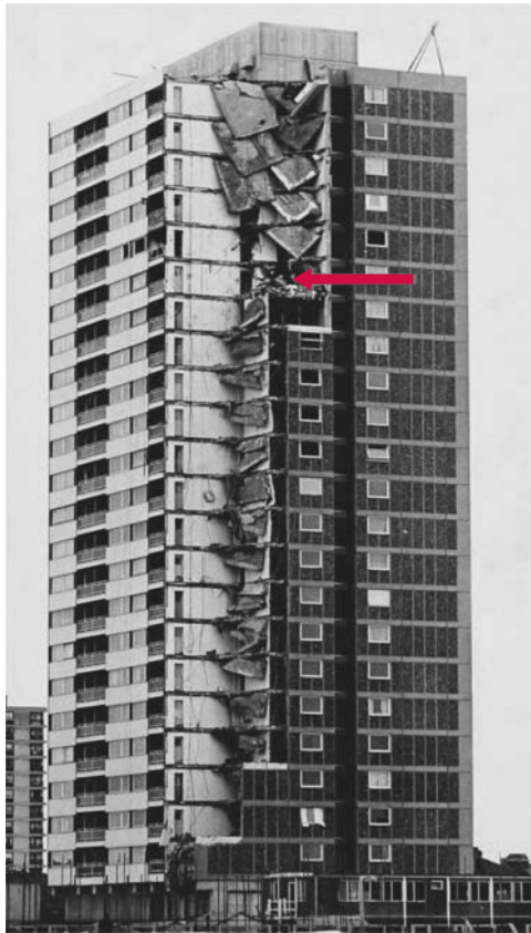
Figure 6.10 Progressive collapse showing point of explosion. (Ronan Point building collapse, May 16, 1968, London. Courtesy of Building Research Establishment.)
