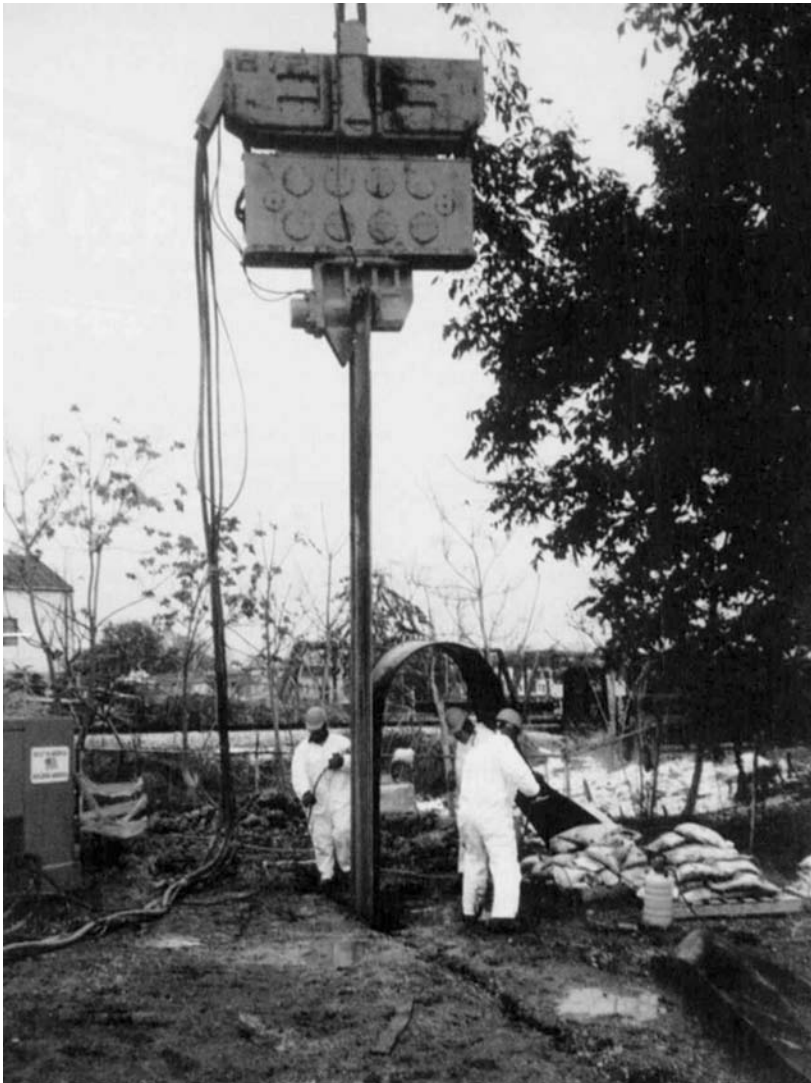
FIGURE 37.20 Installation of HDPE barrier wall utilizing conventional pile driving equipment. (Photo courtesy of Groundwater Control Inc.)
