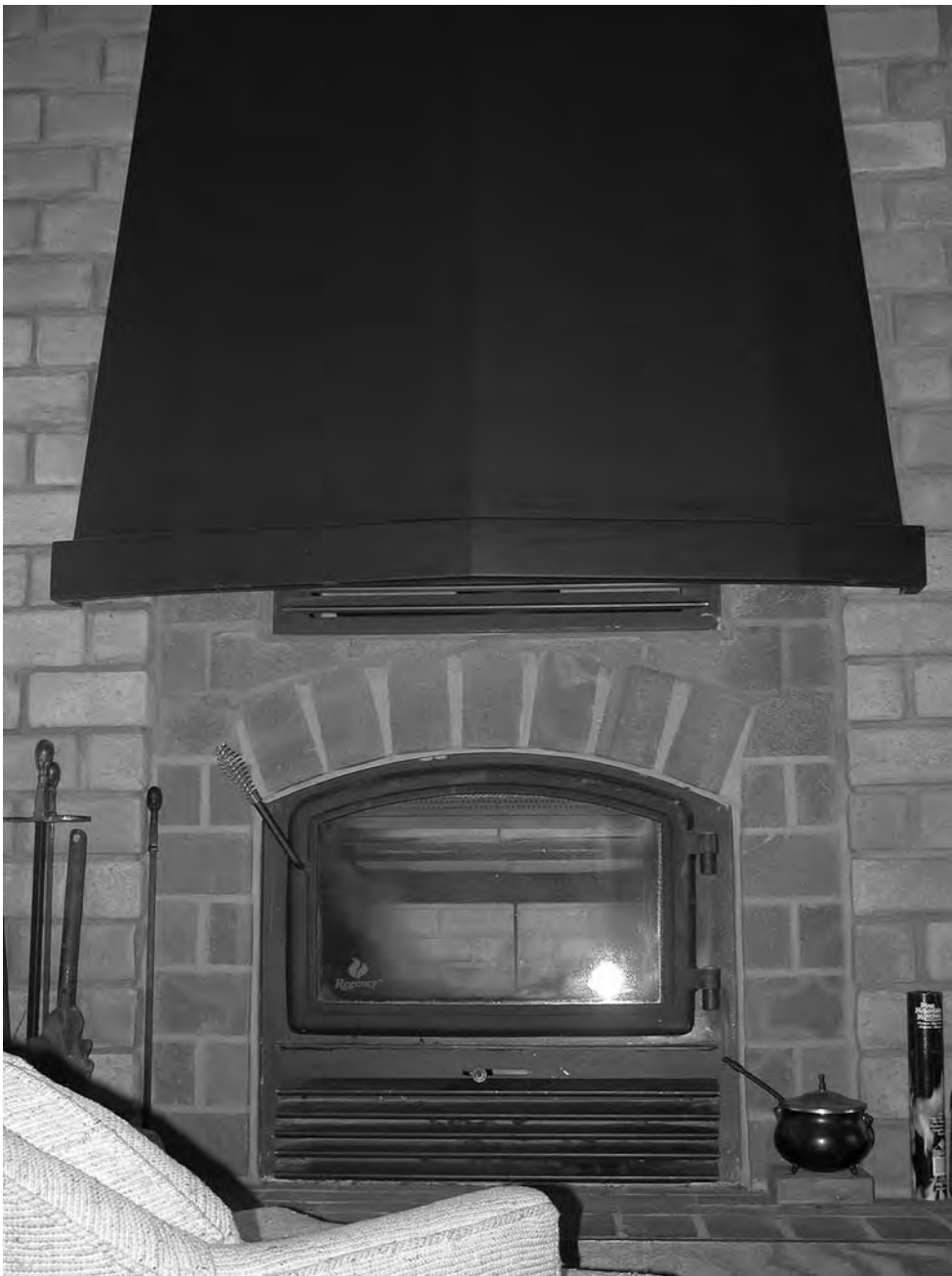
Figure 7.12 Photograph showing heat-producing fireplace.
