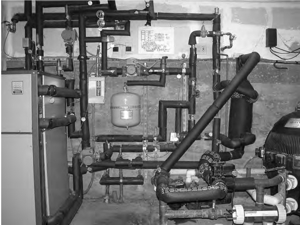
Figure 7.8 Photograph showing the solar piping/control system.
