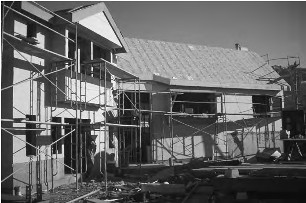
Figure A.8 Completion of the solar roof construction by placement of the R-control panels over the long roof rafters to produce the interior exposed beam vaulted ceiling.
