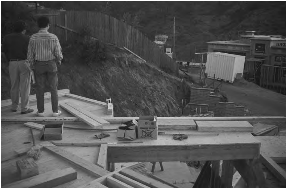
Figure A.2 Architect Ed Nold (left) and general contractor Gary Gerber (right) standing on the start of the second floor on the bridge between the main living/kitchen/dining section to the second floor bedrooms.
