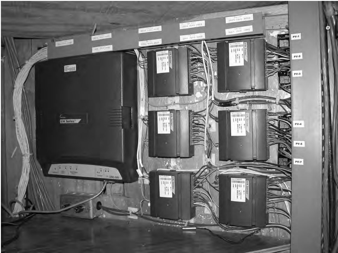
Figure 7.11 Photograph showing control closet hardware.
