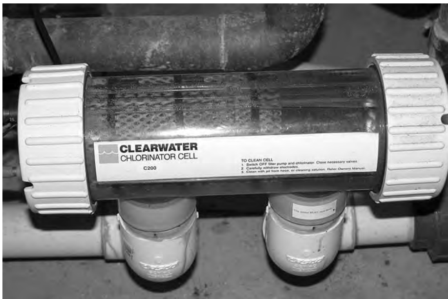
Figure 6.2 Photo of Clearwater solar powered pool chlorinator.
