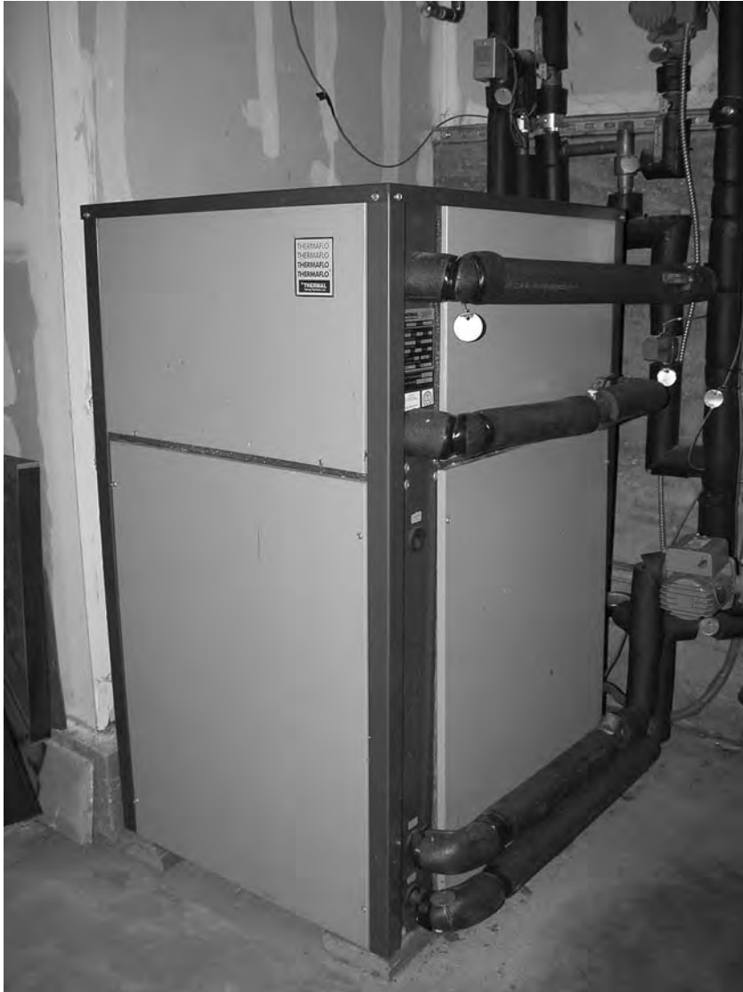
Figure 7.6 Photograph of Berkeley house geothermal heat pump.
