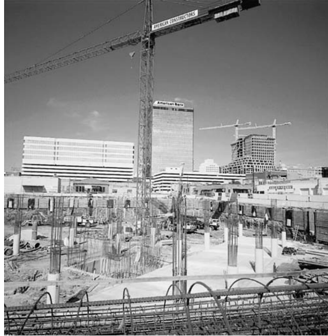
FIGURE 13.1 Concrete piles used for the foundation of a skyscraper. (© Fritz Henle/Photo Researchers.)
