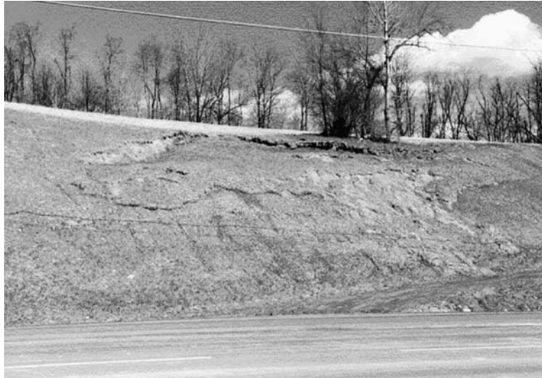
FIGURE 16.1 Slope failure near a roadway. (Courtesy of Todd Mooney.)
