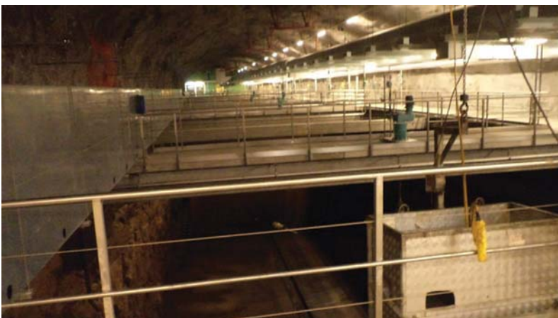
Figure 7.7 Inside view of wastewater treatment tanks located underground at Stockholm.
