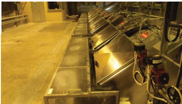
Figure 4.11 Fully automated self-cleaning screen with enclosure.
