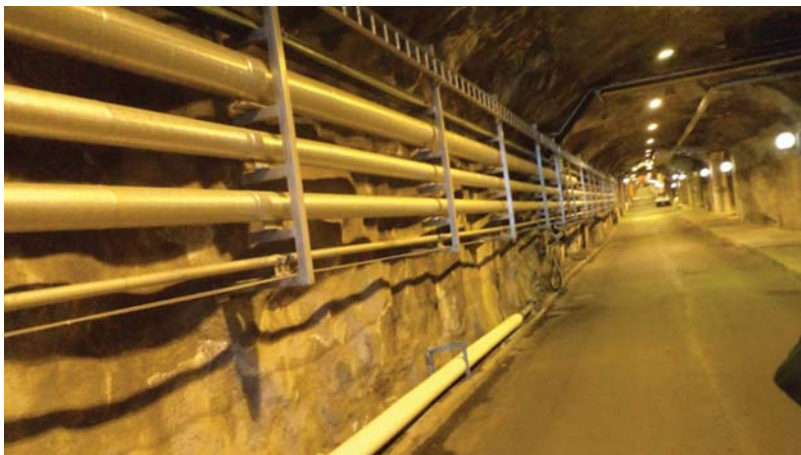
Figure 7.3 Inside view of a wastewater treatment piping located underground in Stockholm.
