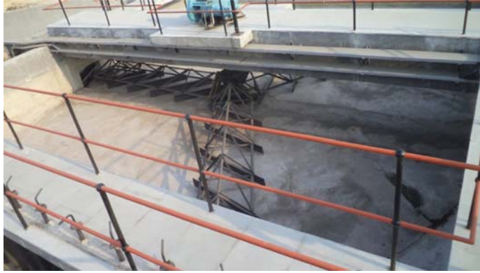
Figure 4.12 A grit-removal chamber with scrapper.
