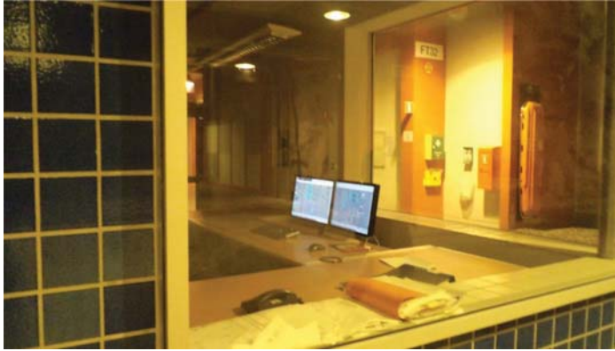
Figure 4.2 Control room of a large sewage treatment plant without process control engineers.
