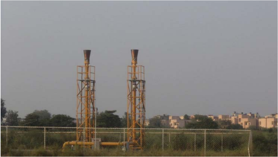
Figure 8.6 Flares for burning methane from wastewater to energy plant.
