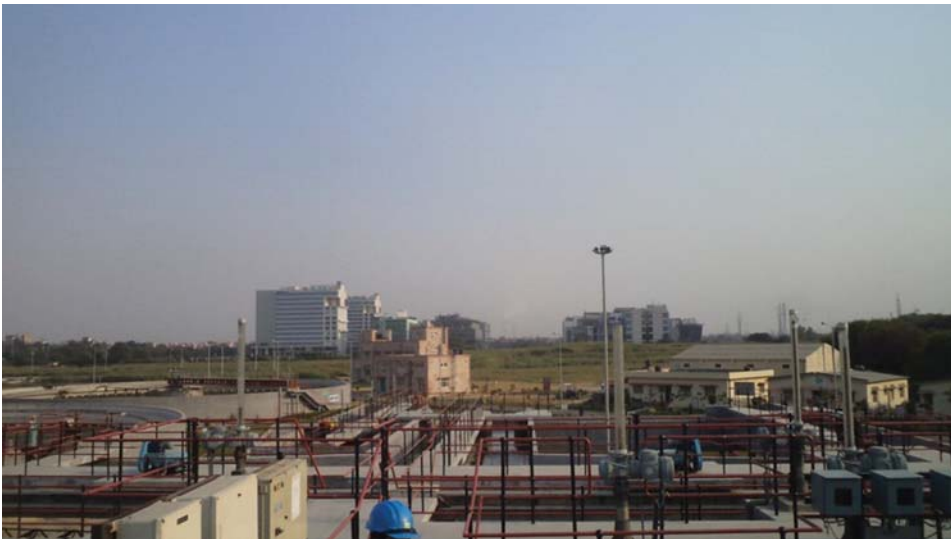
Figure 8.5 Wastewater treatment plant with proper guarding.
