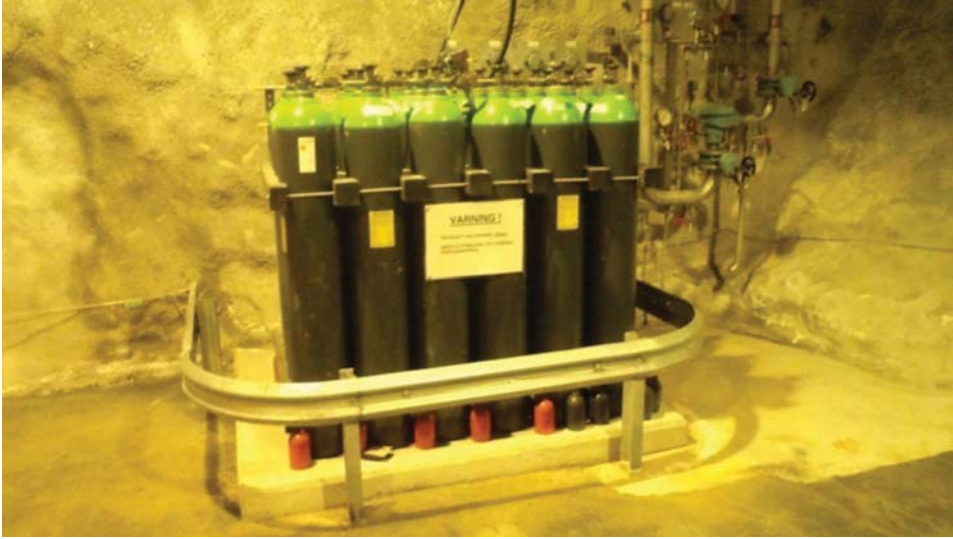
Plate 8.22 Chlorine stored at wastewater treatment plant site.
