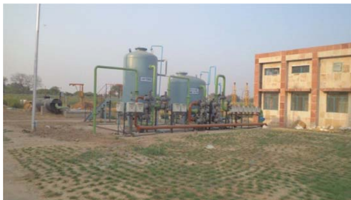
Figure 4.42 View of pressure sand filter and softener.
