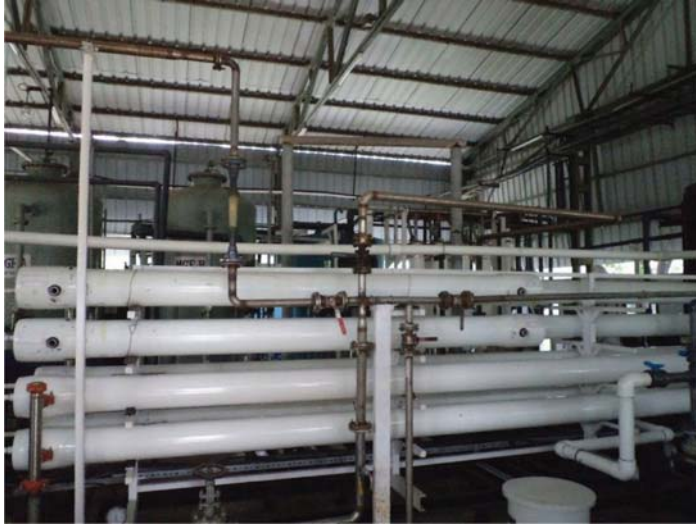
Figure 4.43 Reverse osmosis system.
