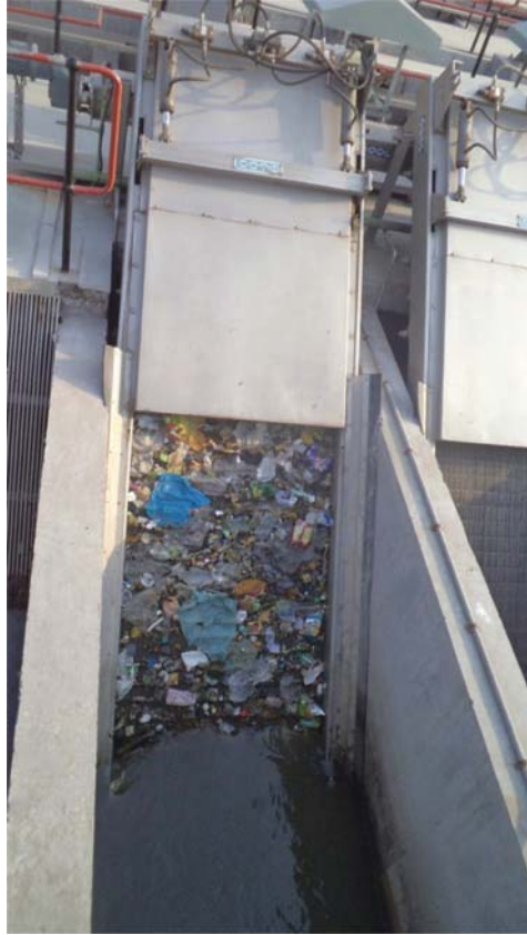
Figure 4.10 Mechanically cleaned screen.
