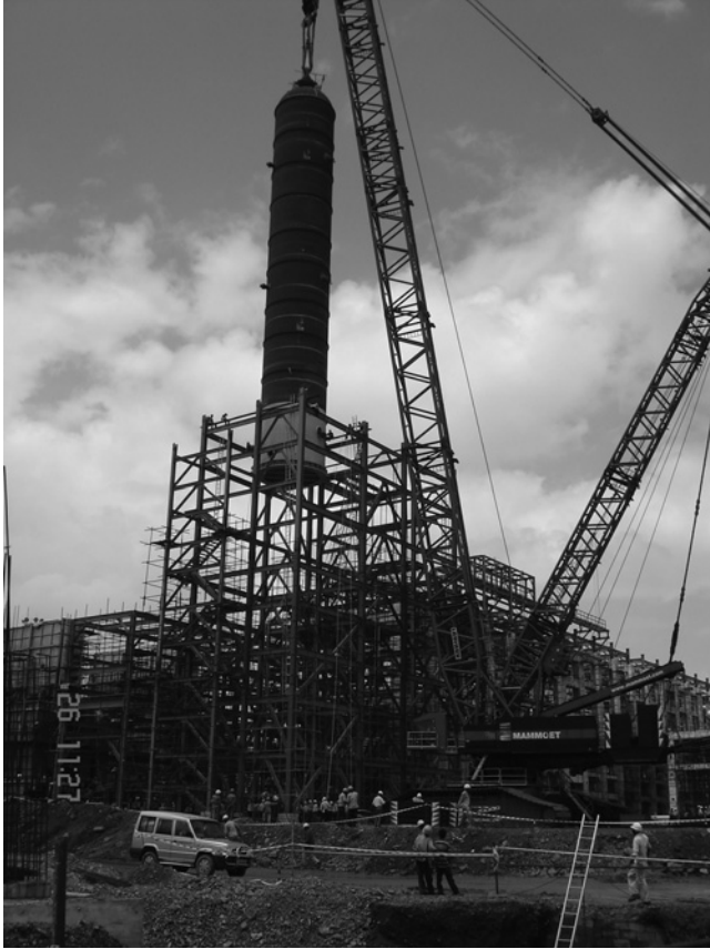
FIGURE 7.23 Thdowering and fnal installation of the hydrocrack er referred to in Figure 7.22 .
