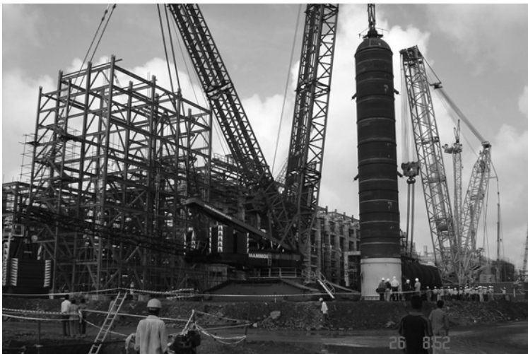
FIGURE 7.22 The actual lifting of the hydrocracker using the top flange lug and tail lugs.
