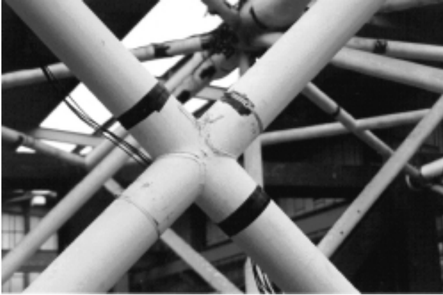
FIGURE 12.22 Tearing in tubular joint.
