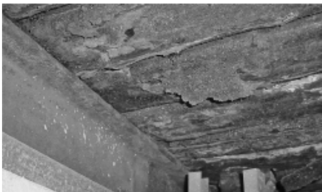
FIGURE 8.12 Corrosion in a corrugated sheet.
