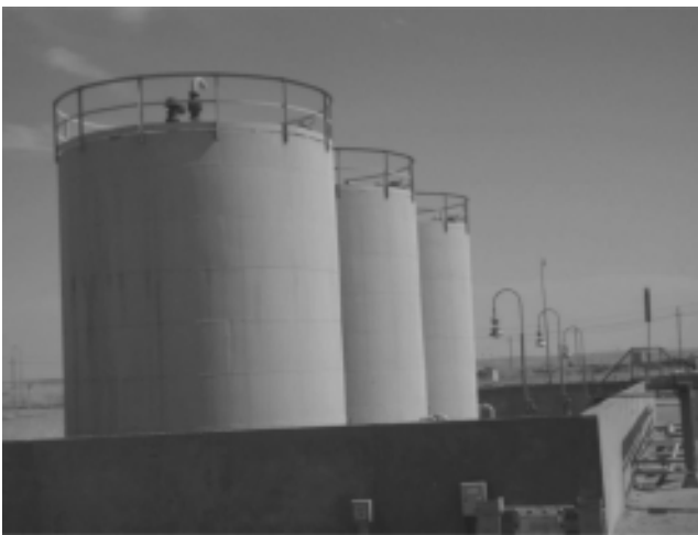
FIGURE 5.16 Condensate tanks inside a dike from retaining the wall.
