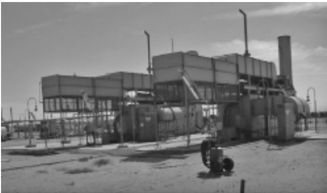
FIGURE 4.2 Gas turbine generator.
