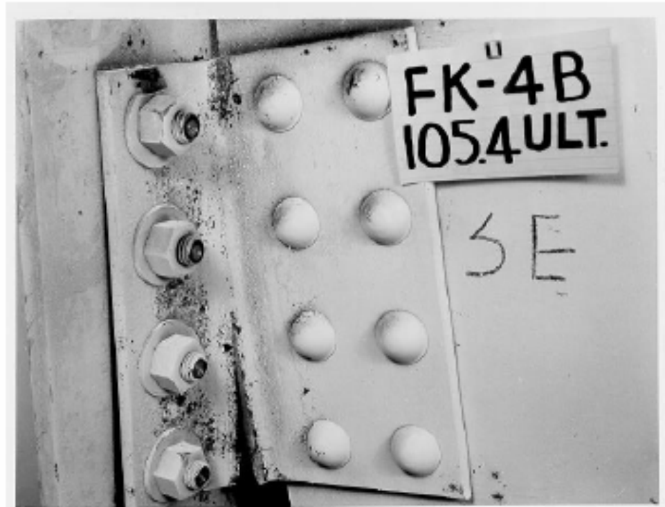
Fig. 18.5. Angle in standard beam connections described in Fig. 18.4. (Courtesy of University of Illinois.)
