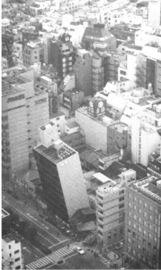
FIGURE 2.41 Nine-story SRC building immediately after the 1995 Kobe Earthquake. (Photo courtesy of NIST; NIST, The January 17, 1995 Hyogoken-Nanbu (Kobe) Earthquake, U.S. NIST, Gaithersburg, MD, 1996.)
