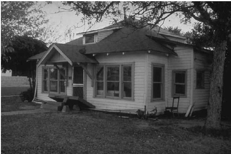
FIGURE 2.34 House that fell from its foundation during the 1971 San Fernando Earthquake. (Photograph courtesy of Steinbrugge Collection, Earthquake Engineering Research Center, University of California, Berkeley.)
