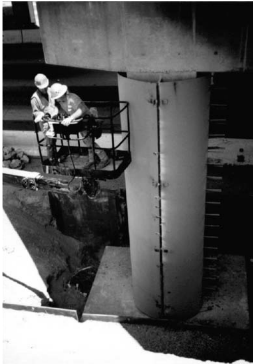
FIGURE 2.89 Steel shell being wrapped around a concrete bridge column to increase its ductility and shear strength.
