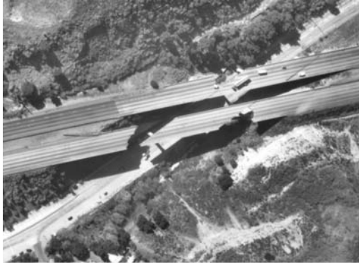
FIGURE 2.43 Damage to Gavin Canyon UC during the 1995 Northridge Earthquake.
