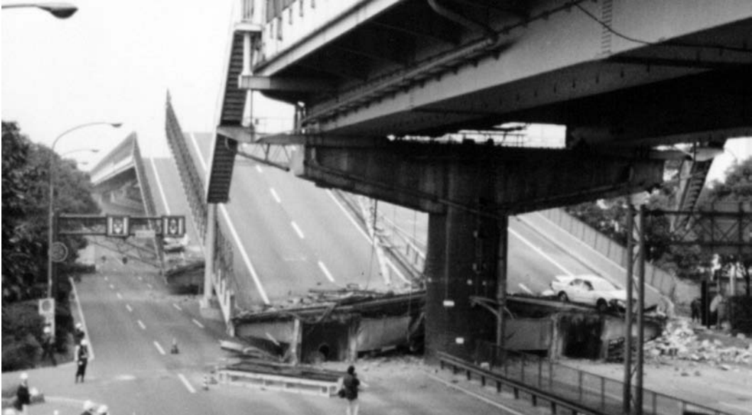
FIGURE 2.56 Superstructure collapse at Spans 40 and 41 on Kobe Route 3.
