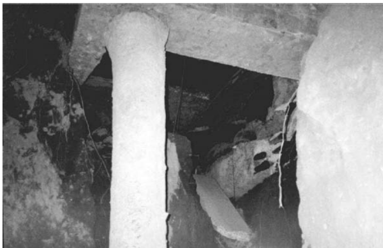
FIGURE 2.69 Washed-out abutment fill caused by water pipe break.
