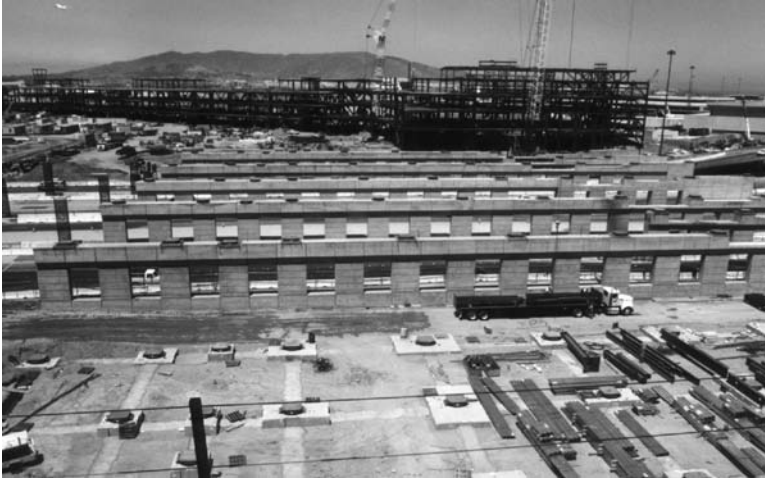
FIGURE 2.78 Layout of foundations and friction pendulum devices for the new San Francisco Airport International Terminal. (Photo courtesy of Earthquake Protection Systems Inc.)
