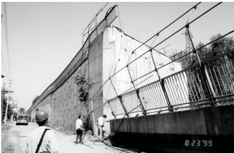
FIGURE 2.73 Mechanically stabilized earth wall continues to support the embankment behind the collapsed Arifiye Overcrossing after the 1999 Kocaeli, Turkey, earthquake.
