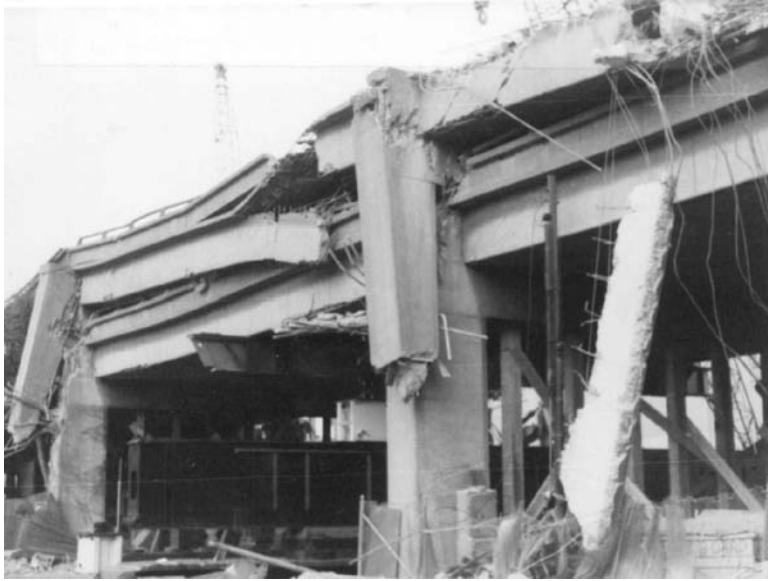
FIGURE 2.28 Damage to Cypress Street Viaduct.
