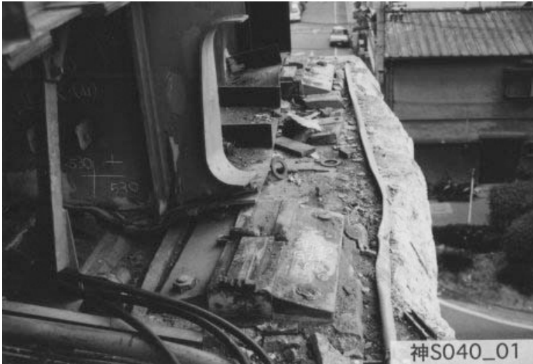
FIGURE 2.58 Broken bearings at Pier 40. (Photo courtesy of Hanshin Expressway Public Corporation.)
