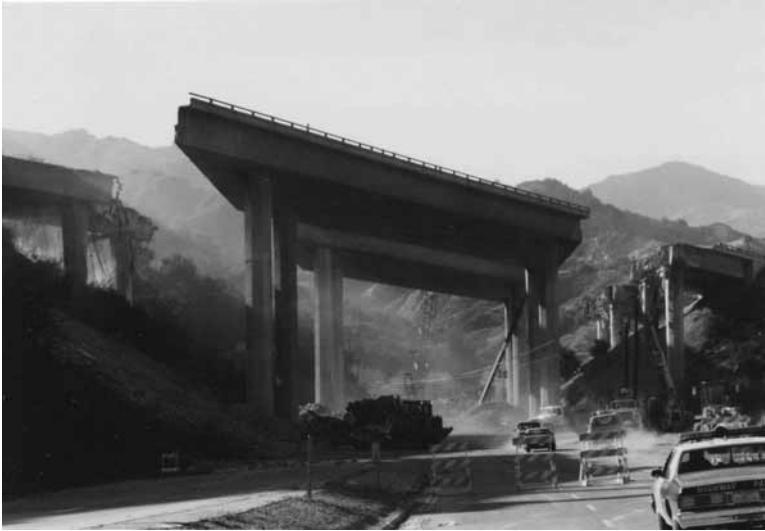
FIGURE 4.2 Collapse of I-5 Gavin Canyon Undercrossing, California, in the 1994 Northridge Earthquake.
