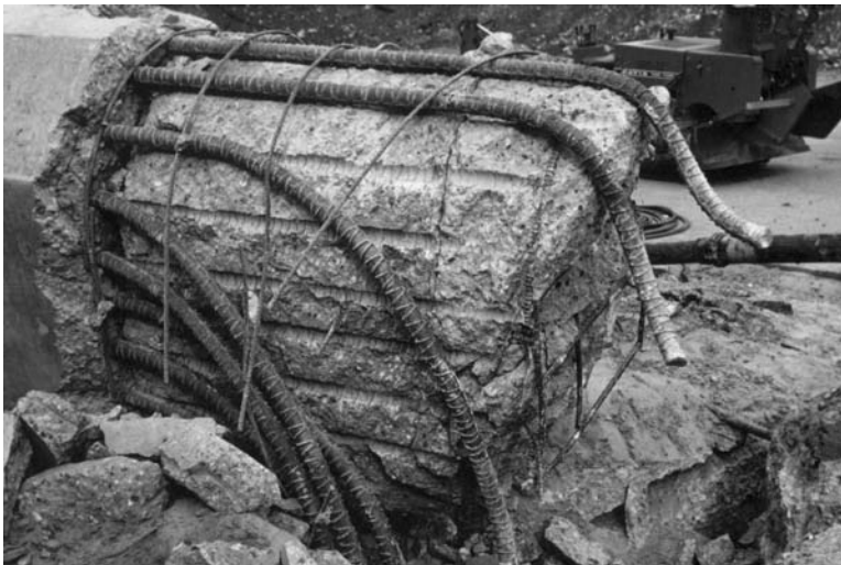
FIGURE 2.36 Failure of column to footing connection.
