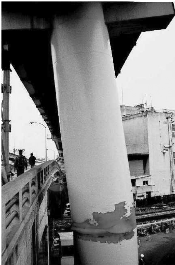
FIGURE 2.54 Pier 585 on Kobe Route 3 during the 1995 Kobe Earthquake. (Photo courtesy of Hanshin Expressway Public Corporation.)
