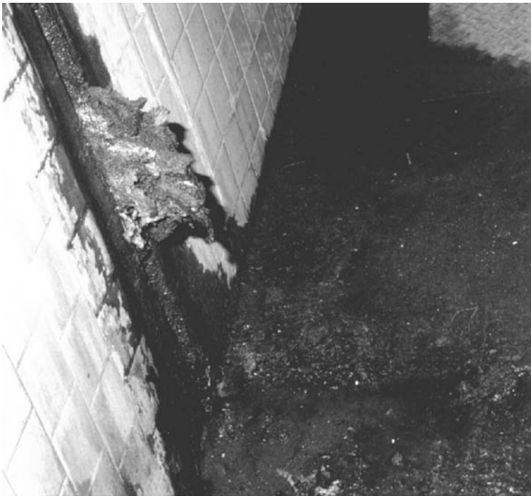
FIGURE 2.11 Liquefaction induced damage to the Webster Street Tube tunnel.
