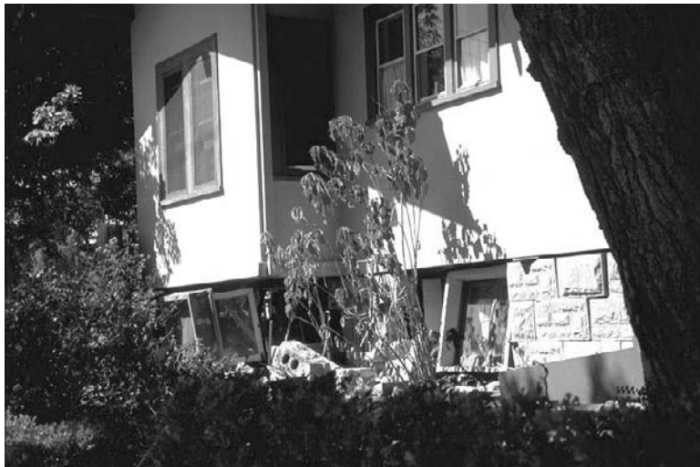
FIGURE 2.32 Failed hollow concrete block foundation during the magnitude 6.0, 1987 Whittier, California, earthquake. (Photo by Karl Steinbrugge. Photo courtesy of Steinbrugge Collection, Earthquake Engineering Research Center, University of California, Berkeley.)
