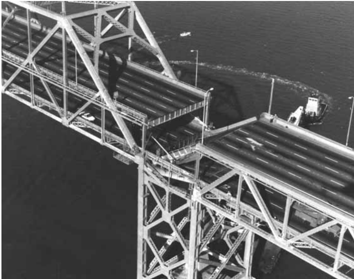
FIGURE 4.1 Collapse of eastern portion of San Francisco-Oakland Bay Bridge in the Loma Prieta Earthquake (courtesy of California Department of Transportation).
