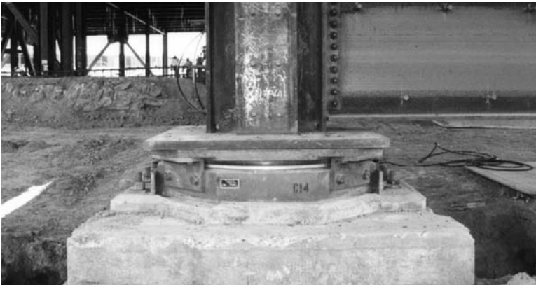
FIGURE 2.79 One of the 267 friction pendulum devices for the new San Francisco Airport International Terminal. (Photo courtesy of Earthquake Protection Systems Inc.)
