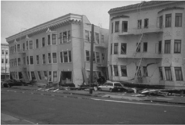
FIGURE 2.37 Soft story collapse in San Francisco during the 1989 Loma Prieta Earthquake. (Photo courtesy of the USGS; The Loma Prieta, USGS, 1998.)
