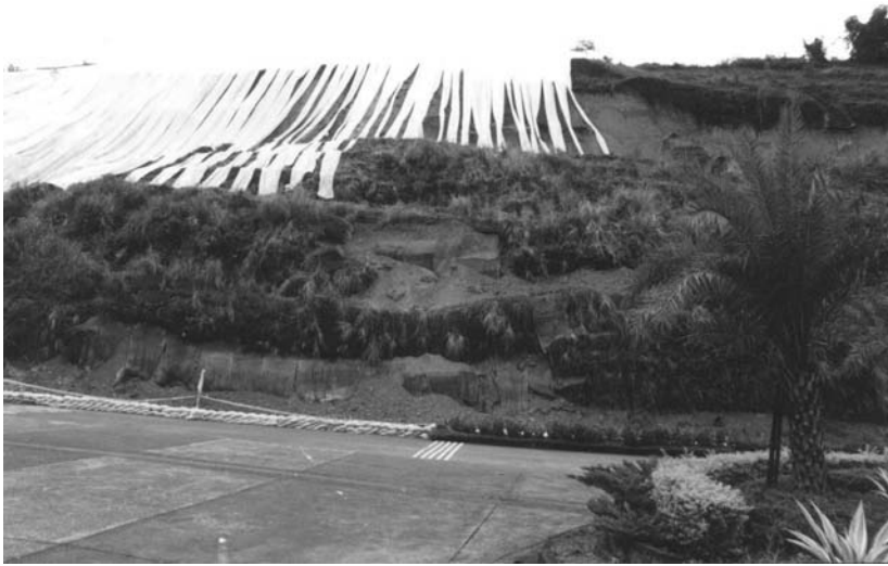
FIGURE 2.15 Fabric retaining wall damaged during the 1999 Ji Ji, Taiwan, earthquake.
