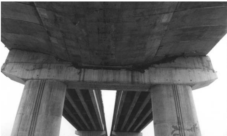
FIGURE 2.45 Damage at end-supports to Ji Lu cable-stayed bridge.
