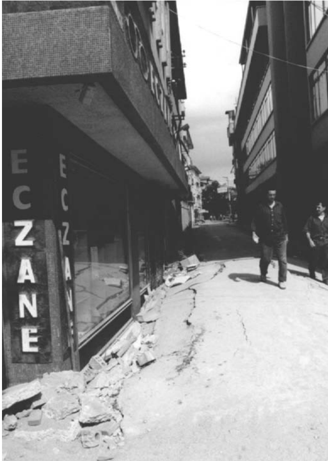
FIGURE 2.6 Settlement of building due to loss of bearing during the 1999 Kocaeli Earthquake.
