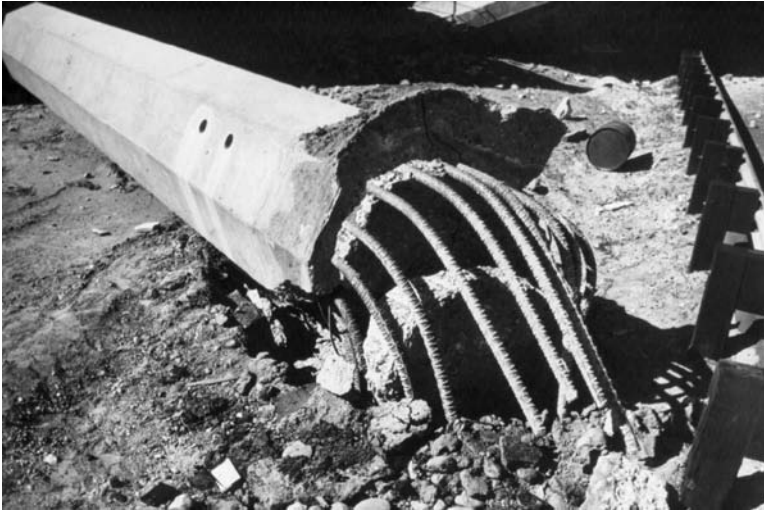
FIGURE 2.35 Failure of column to pile shaft connection.
