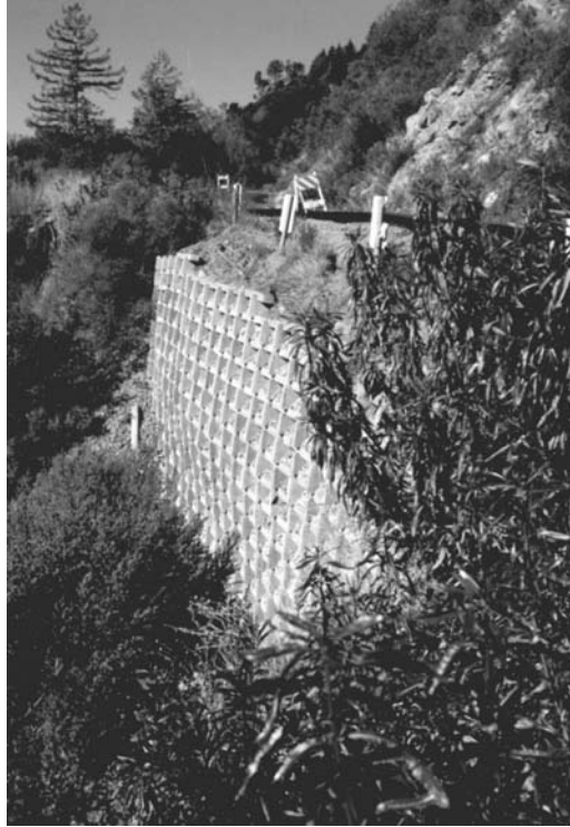
FIGURE 2.74 Crib wall continues to support steeply sloping soil in Santa Cruz after the 1989 Loma Prieta Earthquake. (Photo courtesy of EERI.)
