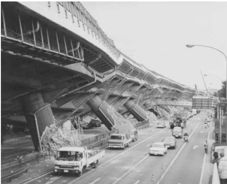
FIGURE 4.3 Collapse of Hanshin Expressway in the 1995 Hyogo-Ken Nanbu Earthquake in Japan (courtesy of Mark Yashinsky).
