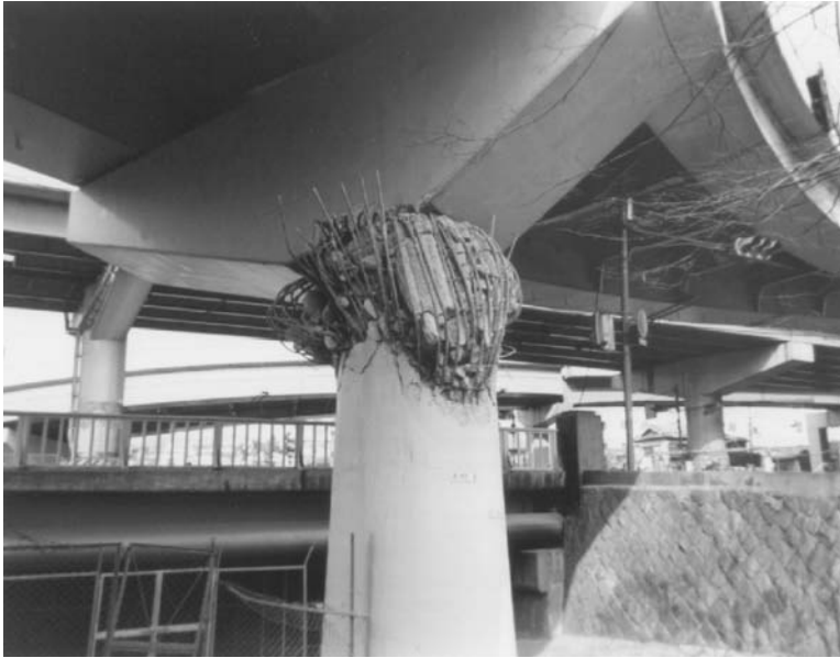
FIGURE 2.46 Column damage to the Minatogawa interchange during the Kobe Earthquake.
