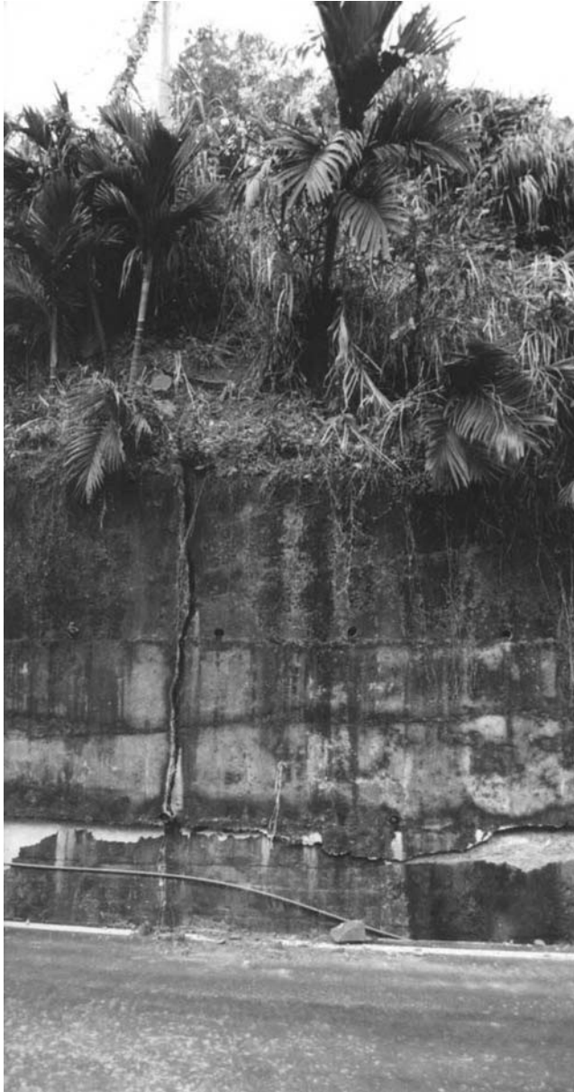
FIGURE 2.14 Gravity retaining wall with shear damage from landslide.
