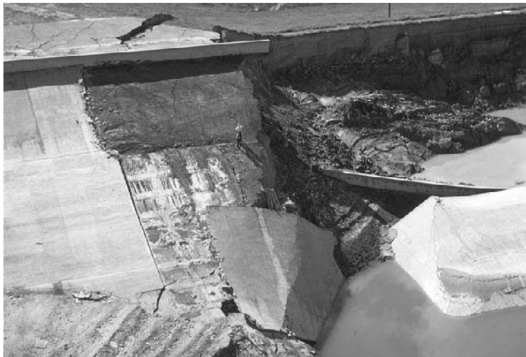
FIGURE 2.22 Closer view of damage to the Lower San Fernando Dam. (Photograph courtesy of Steinbrugge Collection, Earthquake Engineering Research Center, University of California, Berkeley.)
