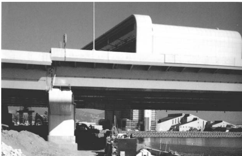
FIGURE 2.7 Liquefaction caused bridge damage during the Kobe Earthquake.
