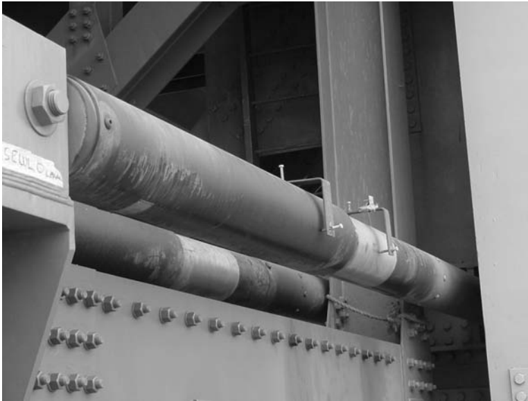
FIGURE 2.88 The Vincent Thomas Bridge retrofit provided gaps between the decks and the towers and also fluid viscous dampers to dissipate energy. (Photo courtesy of Enidine Inc.)
