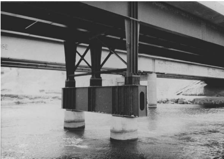
FIGURE 2.86 Lead-rubber isolation bearings on the All American Canal Bridge in California.
