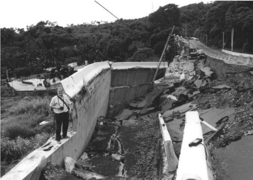
FIGURE 2.13 Gravity retaining wall pushed outward by landslide.
