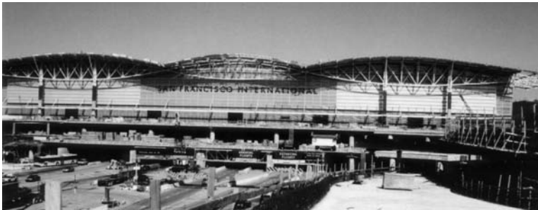
FIGURE 2.77 Construction of the new San Francisco Airport International Terminal. (Photo courtesy of Earthquake Protection Systems Inc.)
