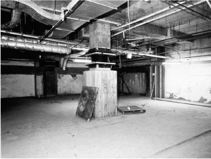
FIGURE 2.85 The concrete columns were cut at midheight and lead-rubber isolation devices were installed. (Photo courtesy of Dynamic Isolation Systems Inc.)
