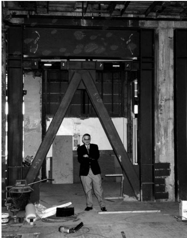
FIGURE 2.83 The steel frames included fluid viscous dampers to reduce the story drift. (Photo courtesy of Marr-Shaffer & Miyamoto, Structural Engineers.)
