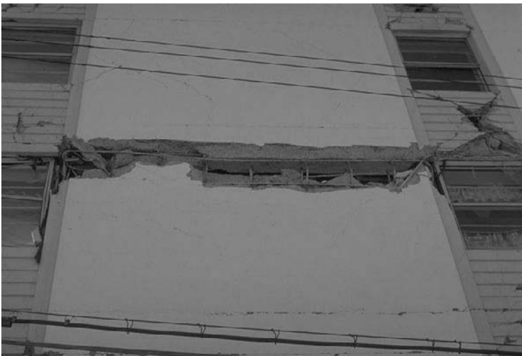
FIGURE 2.49 Damage to north side of Mt. McKinley Apartments. (Photograph by Karl Steinbrugge, Earthquake Engineering Research Center, University of California, Berkeley.)
