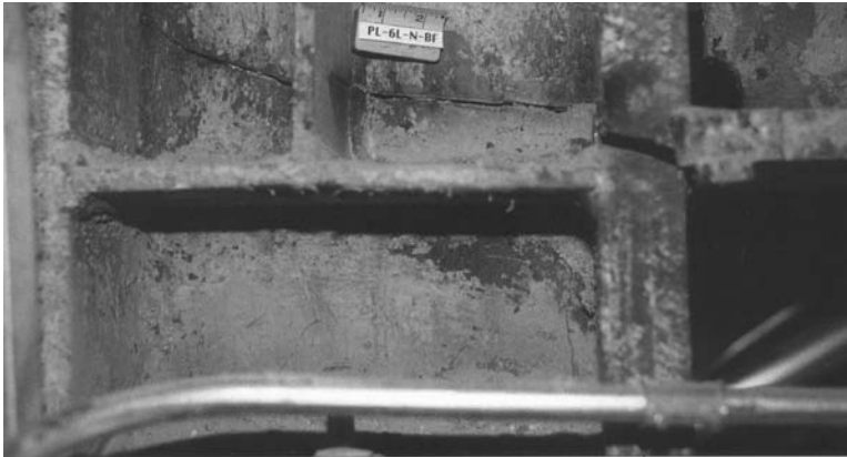
FIGURE 2.60 Steel moment-resisting frame connection after the 1994 Northridge Earthquake. (Photo courtesy of EQE International; EQE, EQE Int. Rev. , Fall, 1–6, 1994.)
