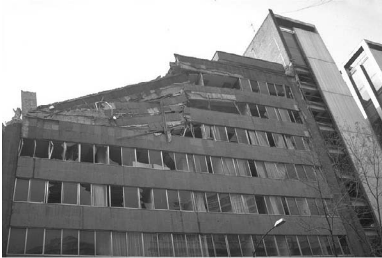
FIGURE 2.31 Damaged 10-story building between the Plaza de la Constitution and Zona Rosa in Mexico City. (Photo by Karl Steinbrugge, from the EERC NISEE Photo Library.)
