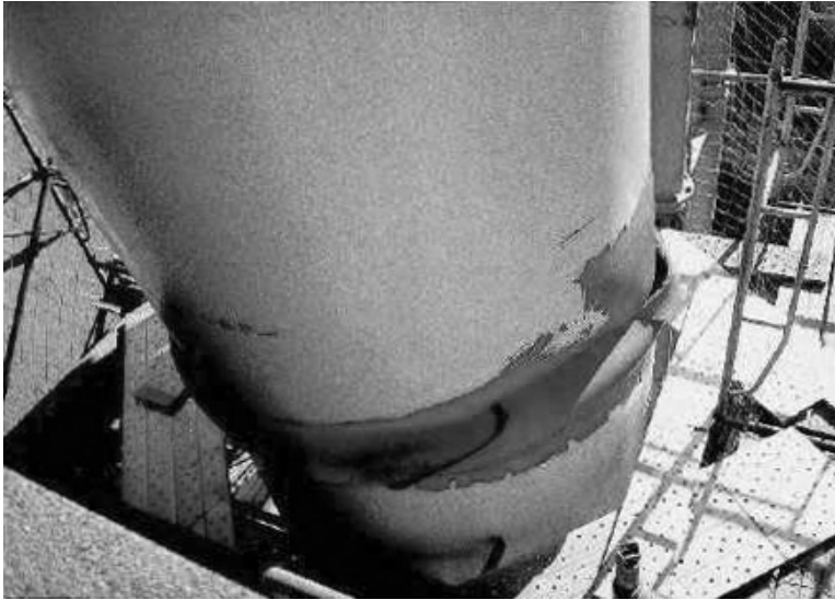
FIGURE 2.55 Torn buckle of steel column on Route 3 after the 1995 Kobe Earthquake. (Photo courtesy of Hanshin Expressway Public Corporation.)
