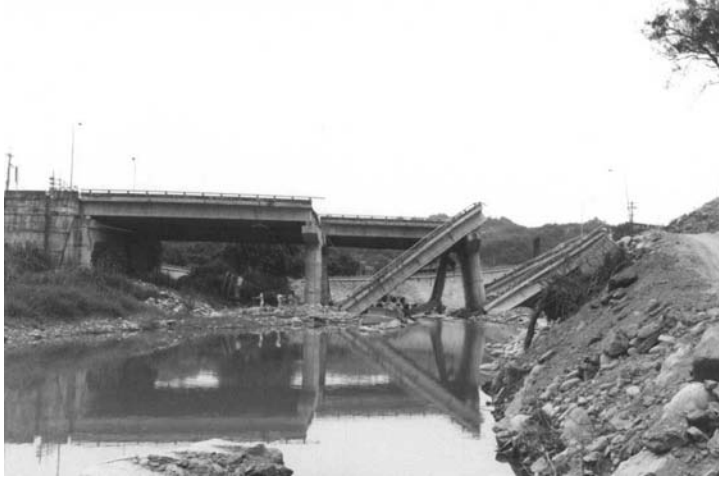
FIGURE 2.19 Collapse of Tsu Wei Bridge due to landslide during the Ji Ji, Taiwan, earthquake.
