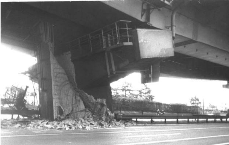
FIGURE 2.51 Shear failure of Pier 150 on Kobe Route 3.
