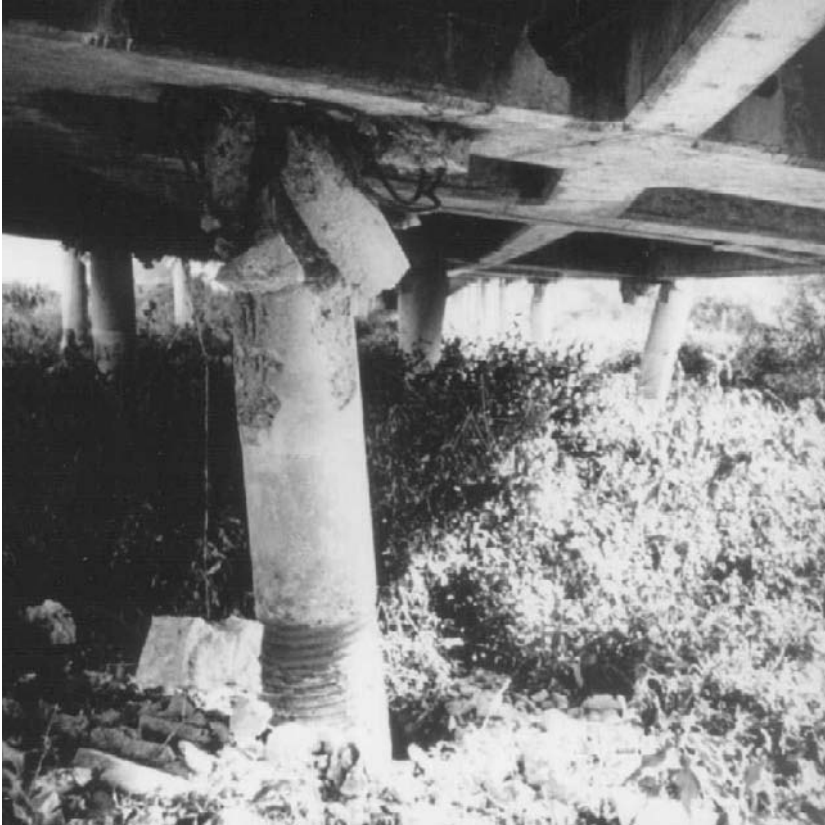
FIGURE 2.25 Broken piles under bridge.
