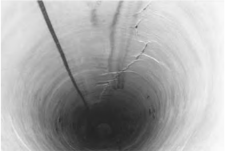
Figure 8.9 The inside of the lined broken rigid pipe test section. The vertical soil pressure is 8700 lb/ft 2 .
