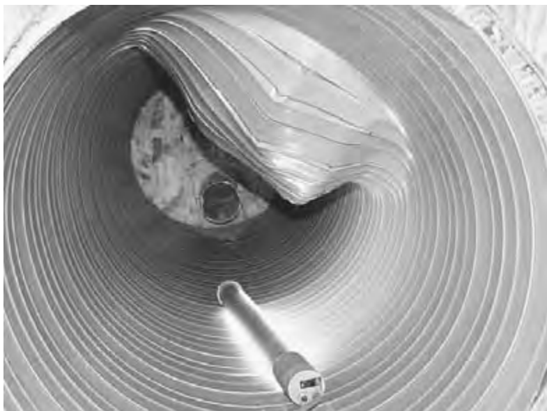
Figure 6.24 Buckling due to 14,000-lb live load over one-half of pipe.
