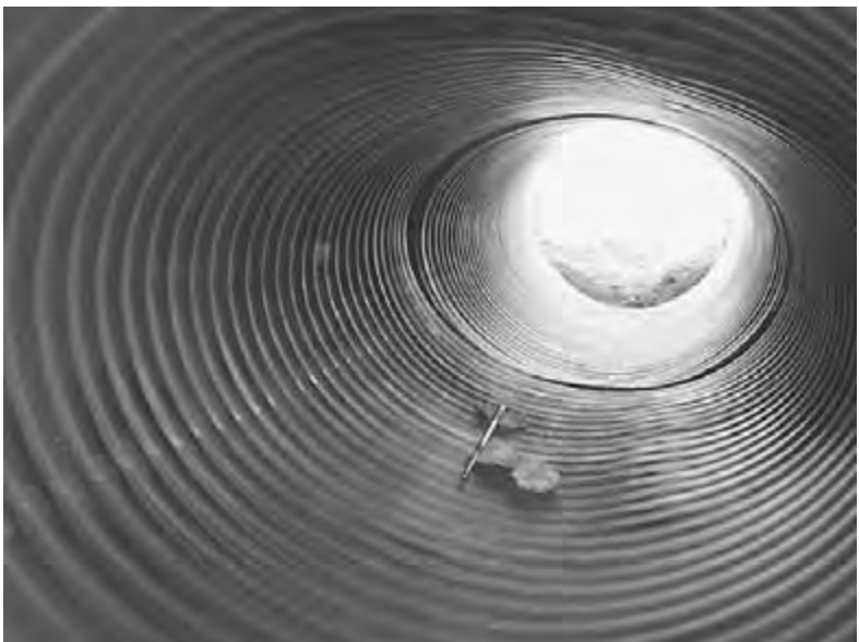
Figure 7.69 Local buckling at 5 o'clock. Density = 77 percent, and load is 46 ft of cover.
