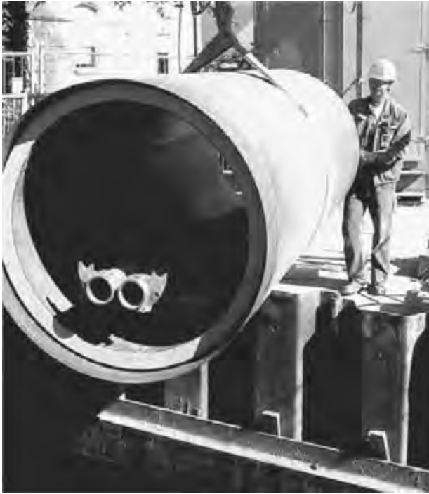
Figure 8.16 Polycrystalline pipe is being placed in the jacking pit. Note prepackaged tubes for supplying fluid to boring machine and removing slurry. (Courtesy of Meyer-Polycrystalline.)
