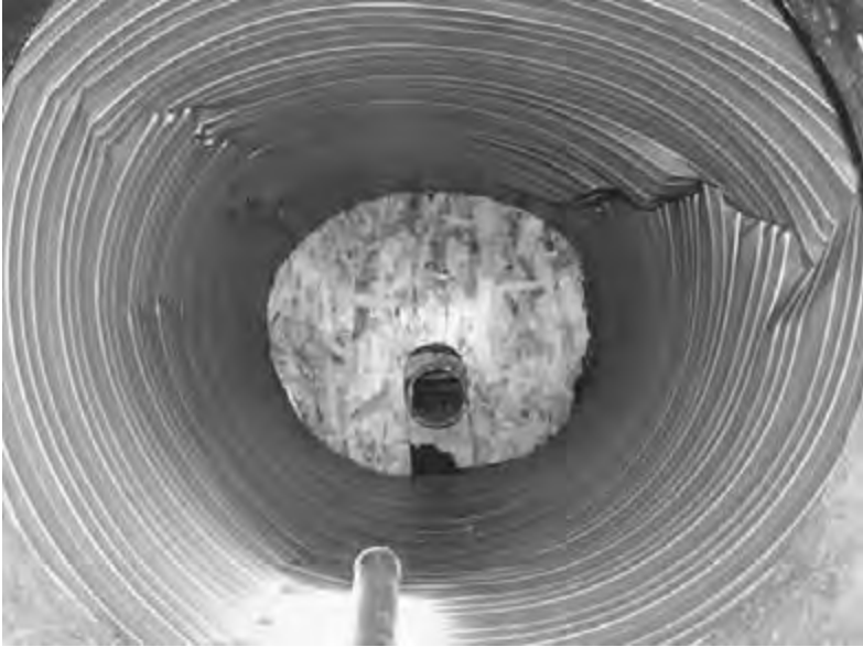
Figure 6.37 Steel-ribbed pipe (24-in diameter) at 43 ft of cover in silty-sand soil at 95 percent density.
