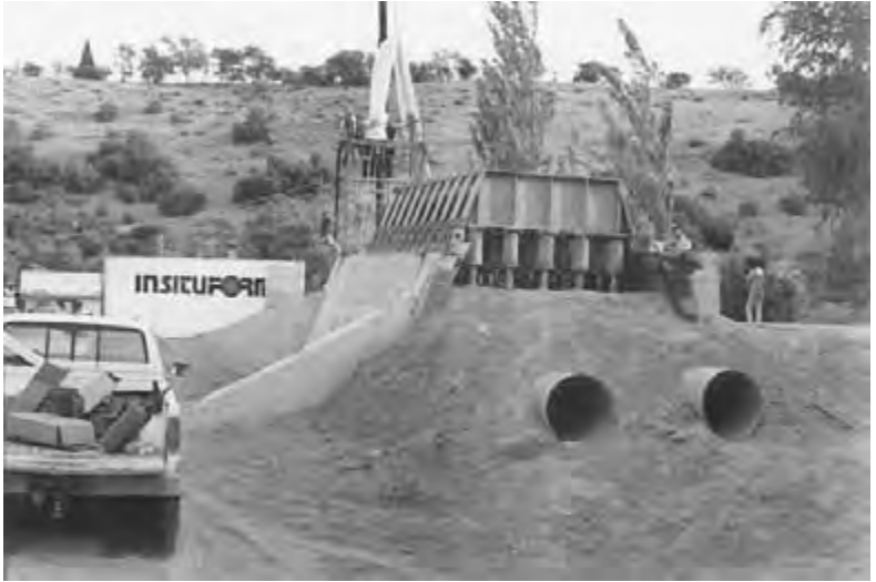
Figure 8.2 Test sections of pipe in place showing the process of inserting the Insituform pipe. The pipes visible are access pipes.
