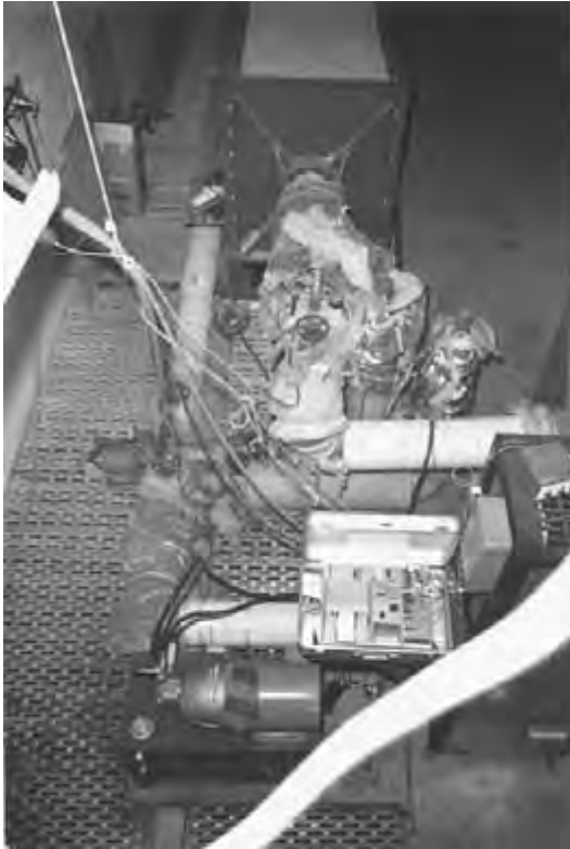
Figure 6.59 Looking down on the heating section located between the two test cells. Note the following: (1) Tops of two 5000-W immersion-type heaters (center right of photo). A third heater is concealed from view. (2) Motor that runs the circulation pump (center left of photo). (3) Insulation applied to external piping to conserve energy.
