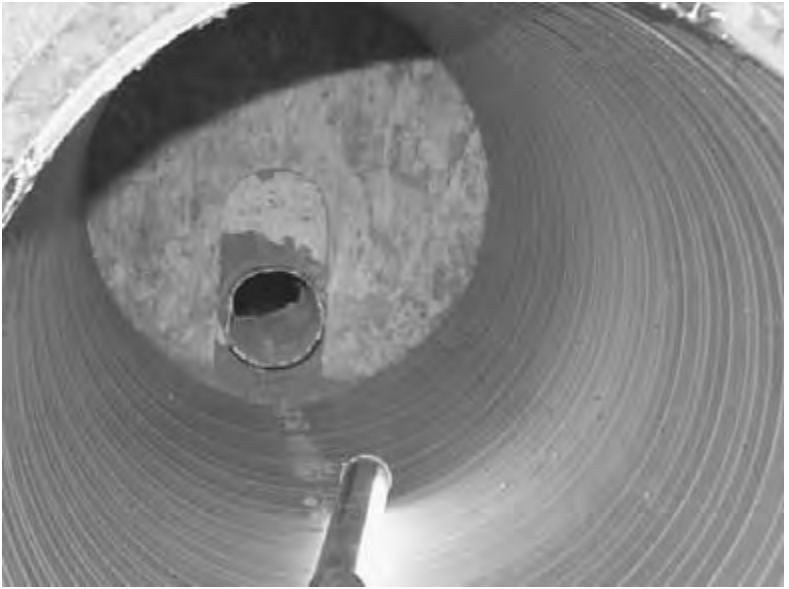
Figure 6.32 A 24-in pipe, with 2 ft of cover, showing no adverse reaction to a 16,000-lb live load.
