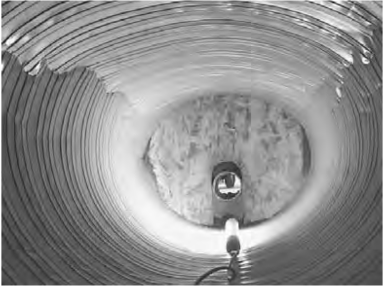
Figure 6.39 Steel-ribbed pipe (24-in diameter) at 49 ft of cover in silty-sand soil at 91 percent density.
