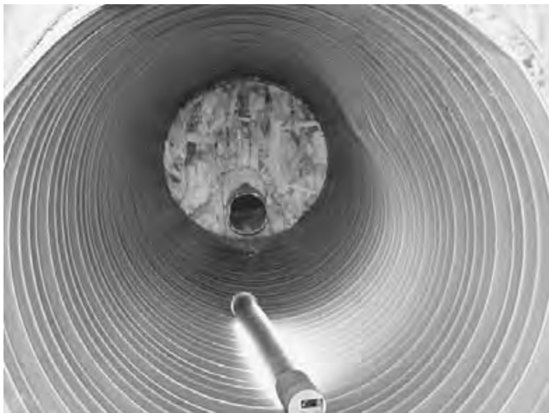
Figure 6.23 Small inversion in sidewall due to 16,000-lb live load adjacent to pipe. Pipe installed with 1 ft of cover.
