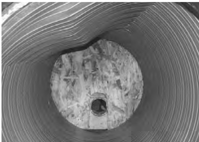
Figure 6.26 Buckled 24-in pipe resulting from a 16,000-lb live load.
