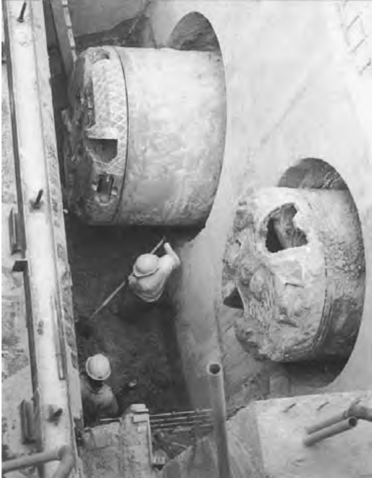
Figure 8.22 Parallel-drive microtunneling machines are right on target as they enter the receiving pit in Dubai. (Courtesy of Herrenknecht GmbH, Germany.)
