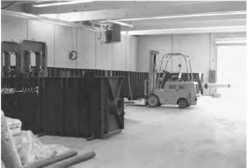
Figure 6.55 Test facility under construction. Foreground: soil load cell; center to rear: water infiltration test cell.
