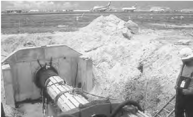
Figure 8.21 Completely unnoticed by the constant air traffic, microtunneling takes place directly under the active runway at the Honolulu International Airport. (Courtesy of Herrenknecht GmbH, Germany.)
