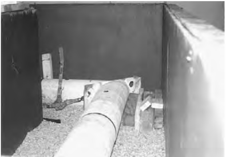
Figure 6.61 Elbow with steel anchor plate before concrete thrust block was cast in corner.
