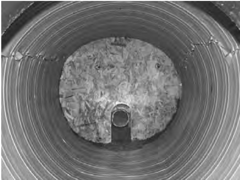
Figure 6.41 Steel-ribbed pipe (30-in diameter) at 60 ft of cover in silty-sand soil at 97 percent density.
