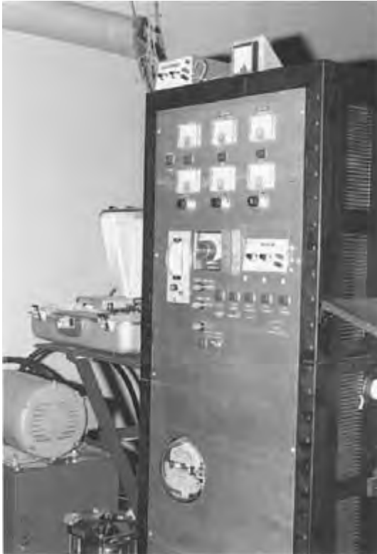
Figure 6.58 System control center with the following features: (1) temperature controller, (2) temperature fail-safe circuits, (3) pressure controls, (4) pressure fail-safe circuits, (5) dual control timer (concealed in photo), (6) flowmeter readout, (7) power meter with digitized output for data system, (8) associated warning lights for system operation. Safety controls were necessary because the system was operated at 500 lb/in 2 and 450° F. An electronically operated pressure relief valve was controlled by the fail-safe circuits. In addition, a manual pressure relief valve was incorporated into the system.
