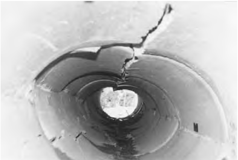
Figure 8.8 The inside of the broken rigid pipe test section after loading to a vertical soil pressure of 8700 \text{ lb/ft}^2 .
