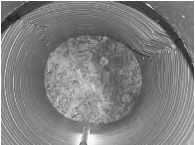
Figure 6.43 Steel-ribbed pipe (30-in diameter) at 42 ft of cover in silty-sand soil at 90 percent density.
