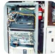
Telecommunication Equipment Cabinet
