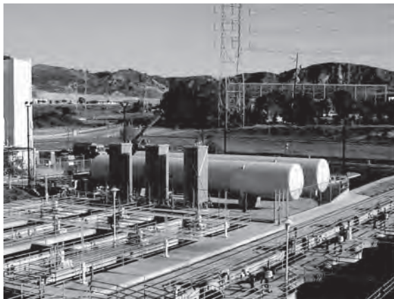
Figure 13-7 Liquid oxygen (LOX) storage container tanks at a large water treatment plant.
