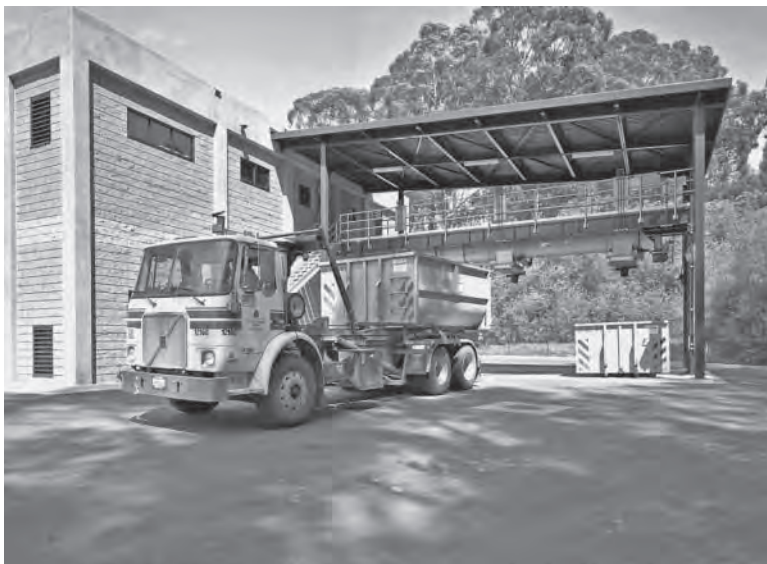
Figure 14-12 Dewatered sludge is placed in large storage containers that are hauled to a landfill, emptied, and returned.
