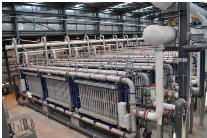
Figure 8-8 Full-scale membrane filtration facility using the pressure-vessel configuration.
