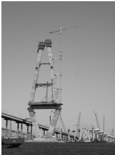
FIGURE 3.8 Cooper River Bridge, Charleston, South Carolina, under construction. (Courtesy of Charles Seim.)
