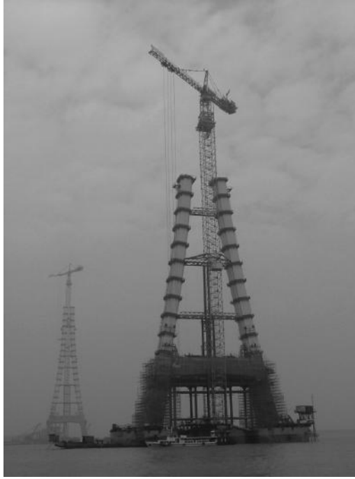
FIGURE 3.12 Third Nanjing Yangtze River Bridge Towers under construction. (Courtesy of Charles Seim.)
