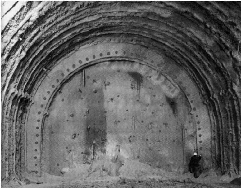
Figure 4-26 Jet grout screen and jet grout columns in the face as ground improvement measures in a tunnel on the new line Bolo- gna – Florence.
