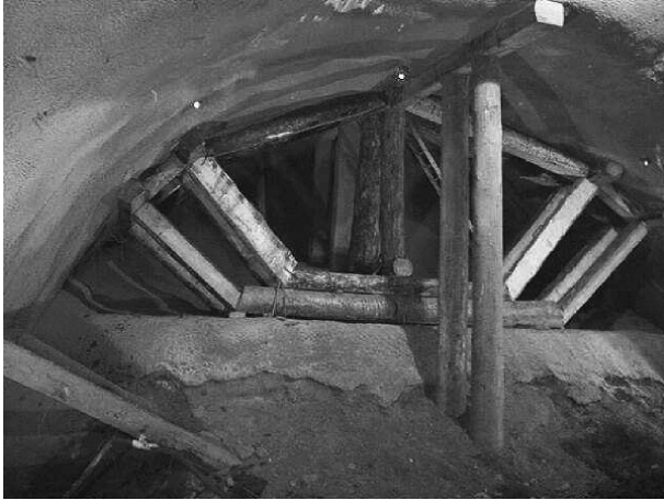
Figure 2-2 Timbering as emergency support after a collapse in the Euerwang Nord Tunnel [136]
