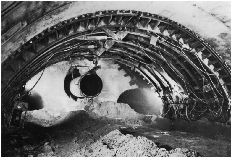
Figure 6-59 Pilot tunnel with ventilation duct to ensure efficient construction ventilation, Milchbuck Tunnel, Zürich
