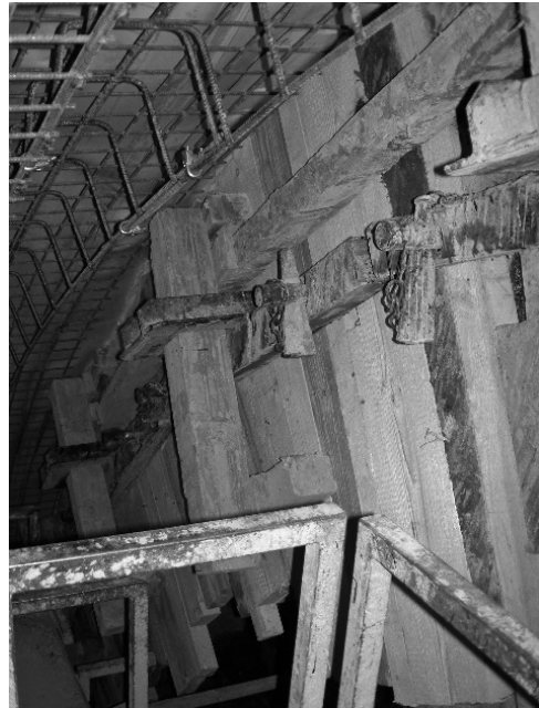
Figure 2-125 Conventional solution for a stopend with wedged formwork panels, Irlahüll Tunnel, new line Nuremberg – Ingolstadt
