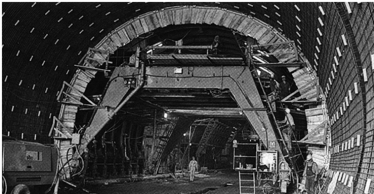
Figure 2-120 Lining formwork unit in use for the construction of the new DB line Hannover - Würzburg (Krieburg Tunnel)
