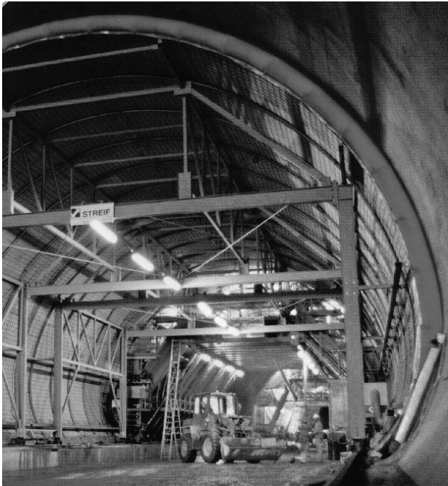
Figure 2-133 Sliding mobile curing unit in the Hellenberg Tunnel on the new line Cologne – Frankfurt [346]
