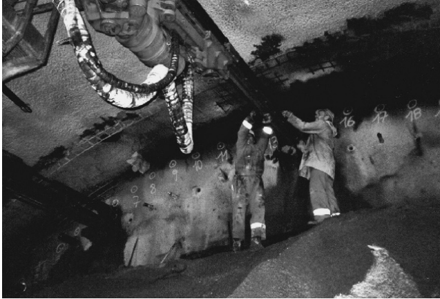
Figure 2-26 Works for the production of a grouted pipe screen using the drilling jumbo in the Irlahüll Tunnel
