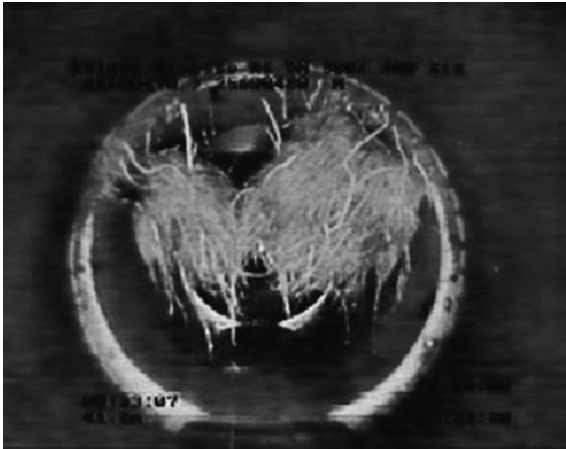
Figure 7-29 Image of roots growing in a pipe from a CCTV survey [349]
