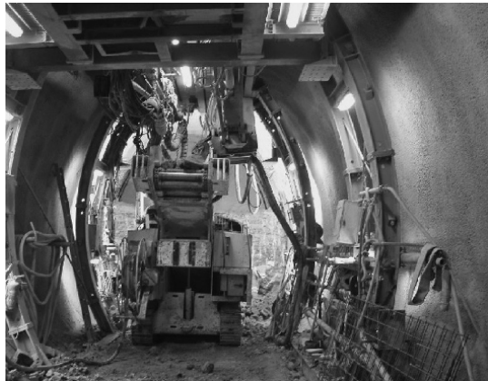
Figure 6-84 GTA Tunnel advance portal in use on the underground railway contract Line 306, Bochum; Beton- und Monierbau [29]
