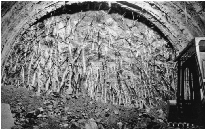
Figure 2-51 Use of glass fibre anchors to support the face in a tunnel for the new line Bologna – Florence
