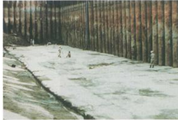
Exposed sea bottom improved by Wet type Deep Mixing Method at the intake of Aioi thermoelectric power station
