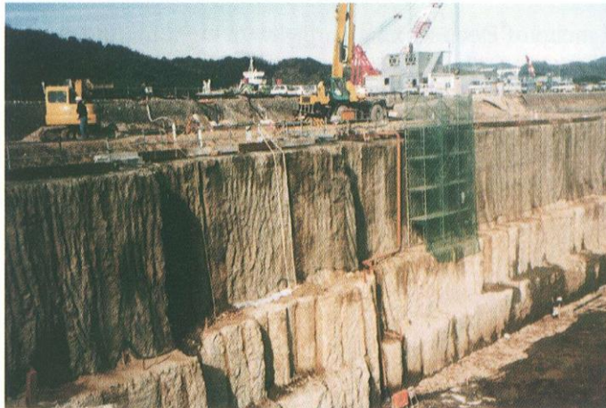
Retaining Wall by Deep Mixing columns - Fly ash cement mixture is used as the stabilizer
