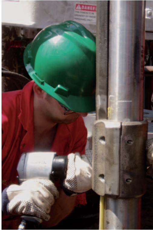
Figure 10.11 Gauge cable and clamp being installed beside tubing (photograph copyright H. Crumpton).
