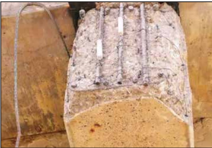
Fig. 43 Deteriorated beam end with concrete removed and embedded galvanic anodes installed
