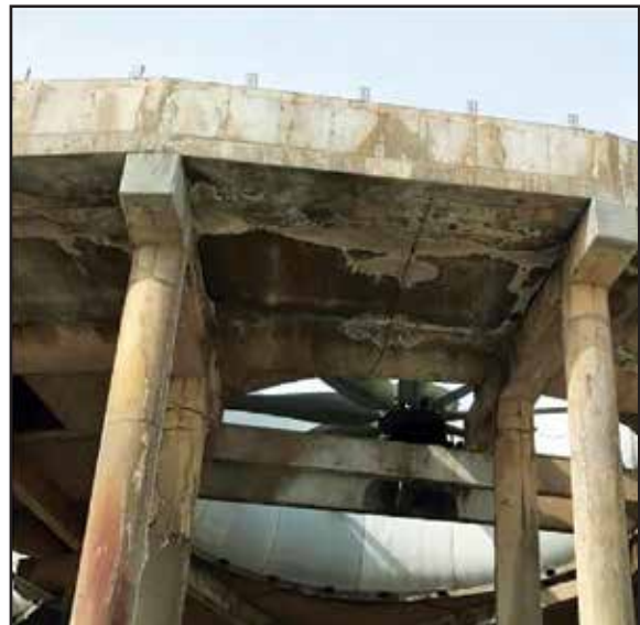
Fig. 37 Leaking joints in precast concrete hot water basin led to deterioration throughout the concrete structure.
