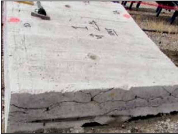
Fig. 14 Saw-cut demolition panel showing delamination cracking at both interior (top) and exterior (bottom) faces.
