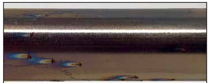
Figure 7. CHO-1 passivation under low hardness conditions of a heat exchanger tube with a heat load.
