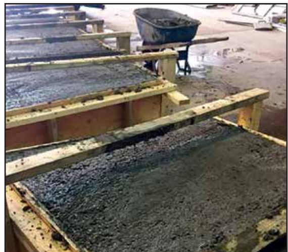
Fig. 46 Precast concrete beams were cast in temporary beds inside the contractor's shop.
