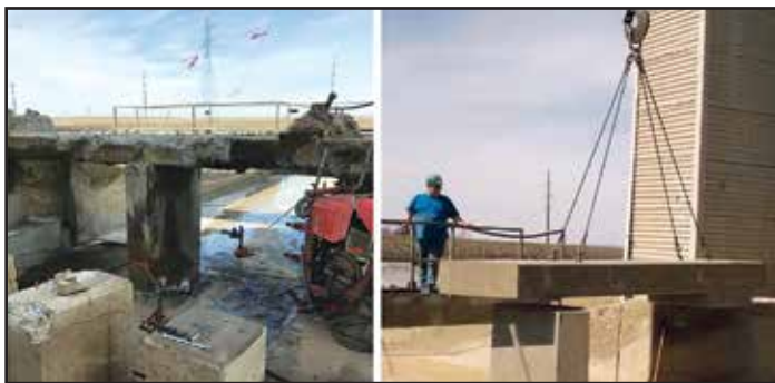
Fig. 48 Concrete repairs at the wall-to-floor cold joint in the cold water basin.
