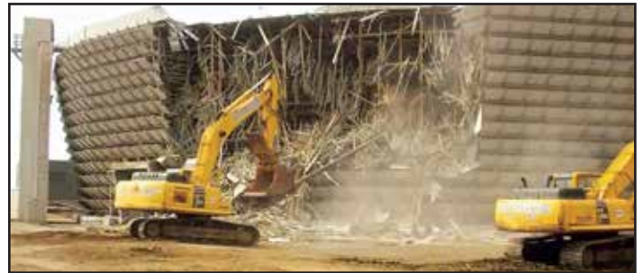
Fig. 36 Demolition of the outer structure of the cooling tower to expose the interior concrete structure.
