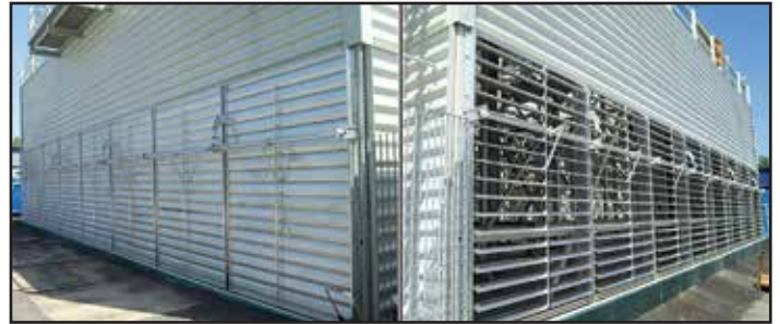
Fig. 2.7: Closed louvers (left) and open louvers (right)
