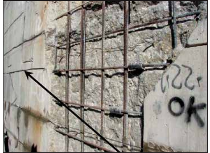
Fig. 17 Partial-depth concrete repair area. Note horizontal saw-cut slots for ICCP ribbon anodes.
