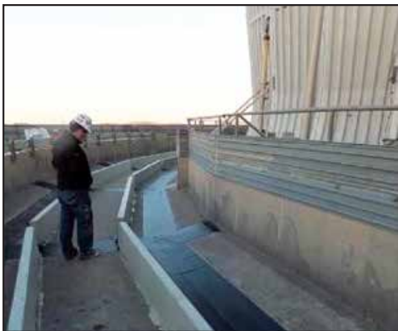
Fig. 38 Completed hot water basin floor repairs including concrete repairs and waterproofing Prepared precast fins with galvanic anodes awaiting new high performance concrete.
