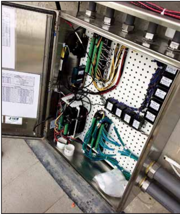
Fig. 34 Rectifier Control Panel Wiring
