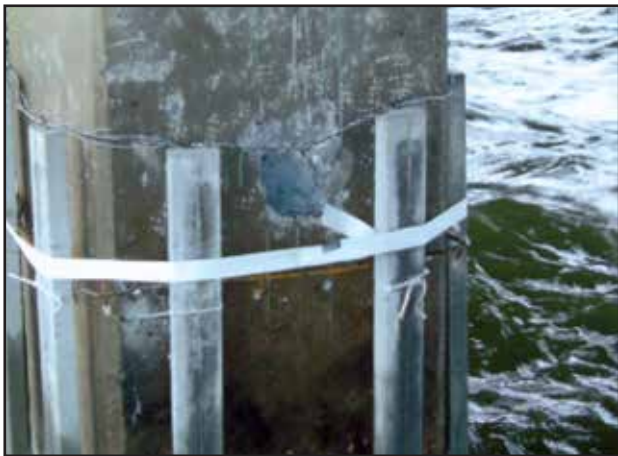
Fig. 11 Galvanic Anode for Marine Application
