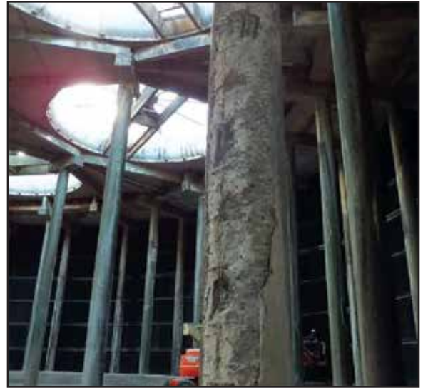
Fig. 44 Example of damaged column under the hot water basin, prior to concrete repair.
