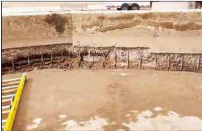
Fig. 47 Severely deteriorated beam was wire cut, removed and replaced with new freeze-thaw resistant precast beams.
