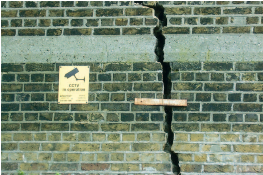
FIG 3.10 London stock brickwork laid in lime mortar to English bond c.1900 and a significant structural fracture which widens to about 75 mm. A crude linear telltale has been fixed over the crack to measure movement. This telltale will indicate the extent of movement over time but it will not tell us which part of the wall is moving relative to the other part, or indeed whether both sections of the wall are moving. A rather more sophisticated method of measurement is needed to confirm precisely what is going on.
