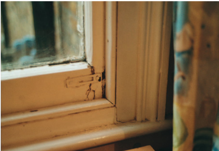
FIG 18.5 Significant expenditure on repairs or replacements of window frames will be needed prior to the next redecoration.
