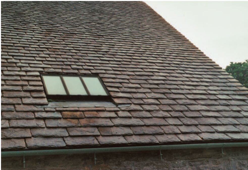
FIG 6.2 Cotswold stone roof with skylight and lead apron. Careful attention to detail is needed if leakage around skylights is to be avoided.
