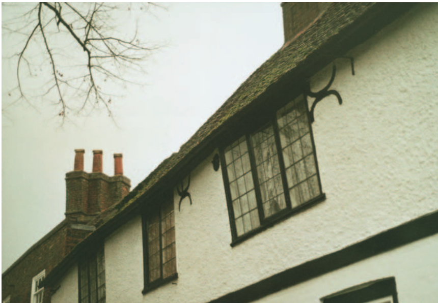
FIG 21.5 The wall around this window leans out and has been restrained by the use of tie bars with the painted tie bar plates used as an added decorative feature. The tie bars will only work if the steel rods are in good order and very firmly secured at the other end.
