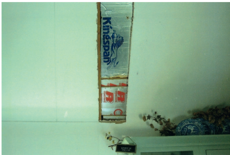
FIG 11.2 A section of plasterboard to a sloping ceiling is removed revealing Kingspan foam insulation panels. Normally, the actual level of insulation above a ceiling cannot be confirmed in these circumstances because there is no access behind. So, the computer program used to provide an energy rating makes certain assumptions based upon the age of the property and the Building Regulations applicable at the time it was built. This presupposes, of course, that the property is correctly dated and that the builders complied with the Regulations.
