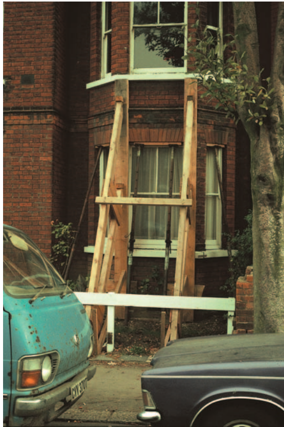
FIG 4.2 Raking shores used to support bay suffering from subsidence pending repair. Note the tree.
