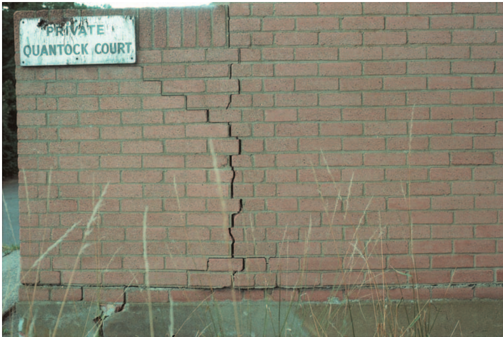
FIG 3.5 A bulge fracture due to compression not related to foundations.
