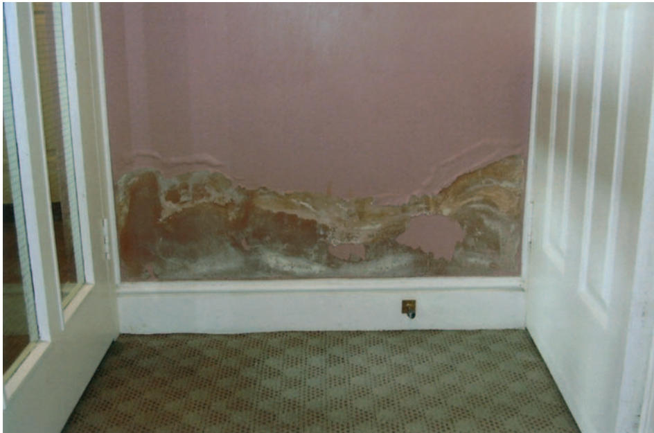
FIG 4.5 Rising damp due to failure of the damp-proof courses will result not only in high readings from a moisture meter but also invisible deterioration to the plaster and decorations. If you cannot see it then it is probably not rising damp. Obviously, there is a problem here which will require investigation, treatment and replastering using a special plaster mix. The condition of any adjacent areas will also need to be checked, especially any timber floors.
