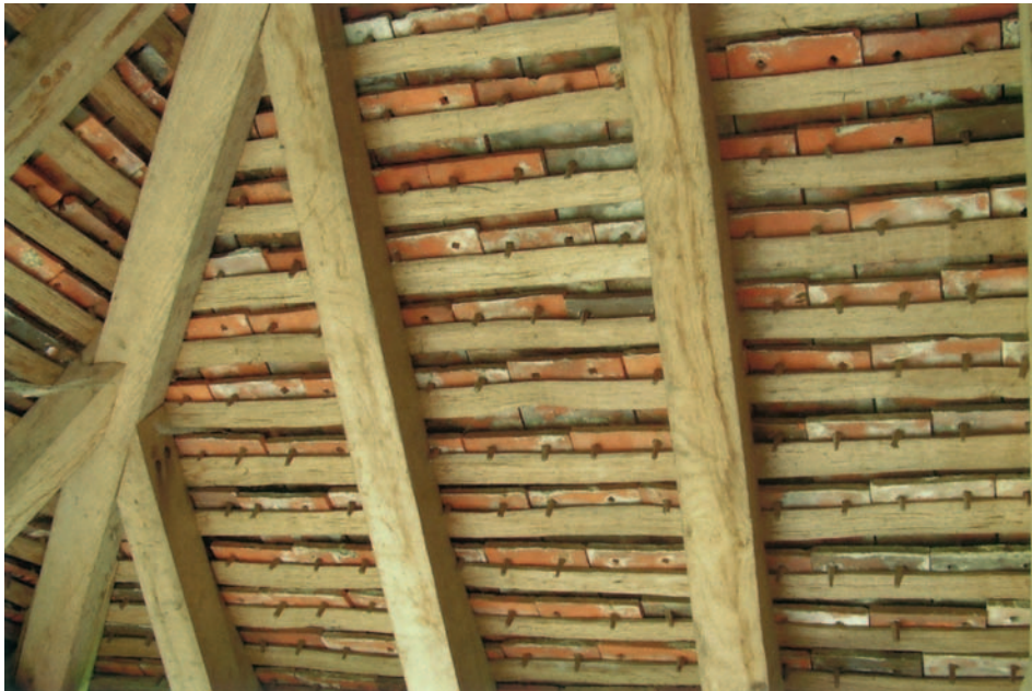
FIG 6.1 Double lap plain clay tiles held in place using traditional wooden pegs on battens with no underfelt. Pegs may rot or shrink causing them to fall out – as has happened to some here – then tiles slip. Tiles can be replaced and, if there is no underfelt, new pegs inserted from beneath, although then the pegs will taper the wrong way and need to be pinned to the battens. This type of tile was gradually superseded in the 19th century by plain tiles with nibs to hold the tiles on the battens. These plain tiles with nibs remain very popular today in both traditional clay and modern concrete form and incorporate nail holes just below the nibs so that they can also be nailed to the battens for an even more secure fixing.
