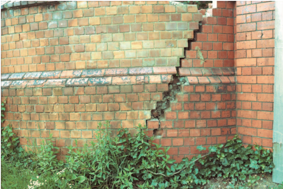
FIG 3.11 Settlement or subsidence. The crack widens with height.
