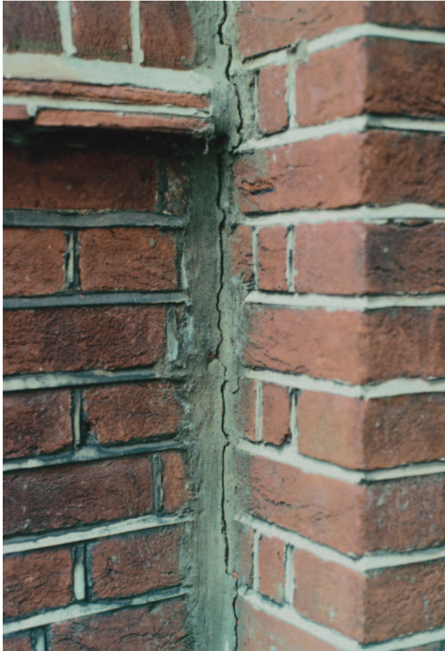
FIG 3.4 This settlement fracture has been poorly repaired and opened up again indicating continuing movement.
