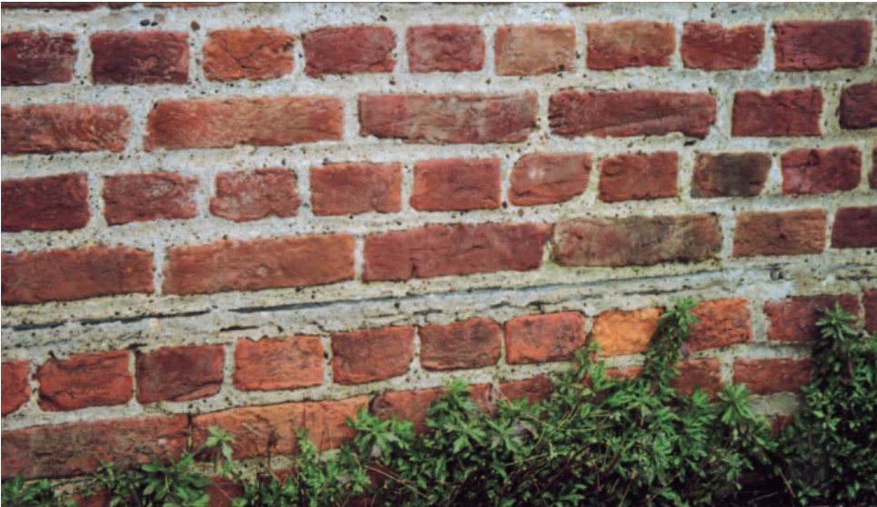
FIG 4.18 Hand-made red facing bricks set in lime mortar to English Bond with a two-course slate damp-proof course. Good ground clearance below the damp-proof course.
