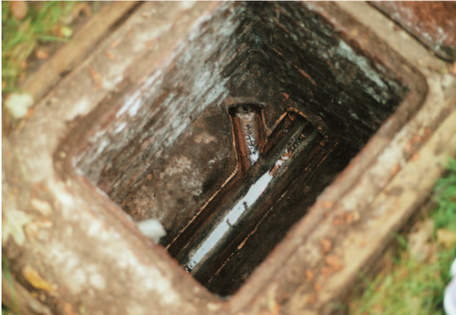
FIG 18.8 One hundred year old drains. Drain flow satisfactory.
