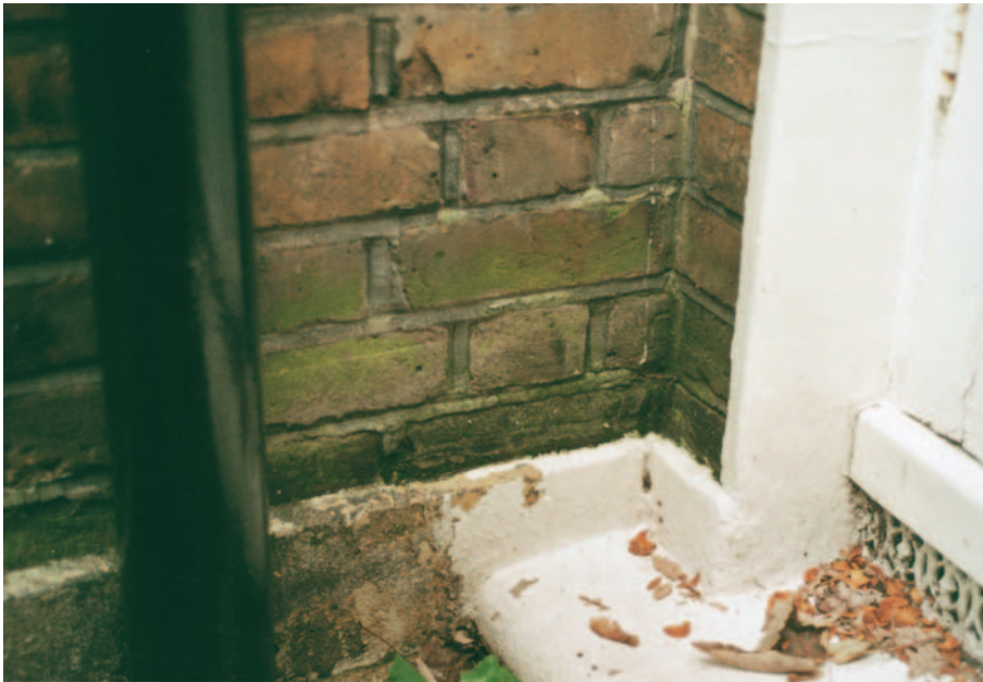
FIG 18.6 Green algae and moss growing at the base of a wall due to gutter splash.
