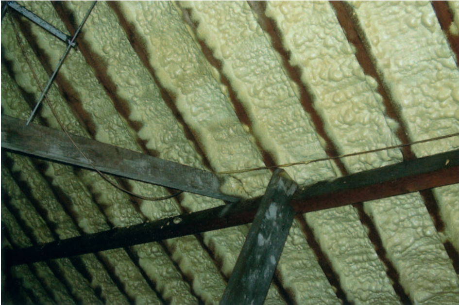
FIG 6.4 Homeowners will sometimes be encouraged by a salesman to have sprayed foam insulation applied from within the roofspace under the tiles and battens between the rafters. I do not recommend this as the timbers cannot breathe, and if they become damp, rotten battens and rafters may result. A roof needing this type of treatment is probably due for recovering with tiles, battens and sarking felt, incorporating ventilation. The best place for insulation is directly over the ceilings between the joists.
