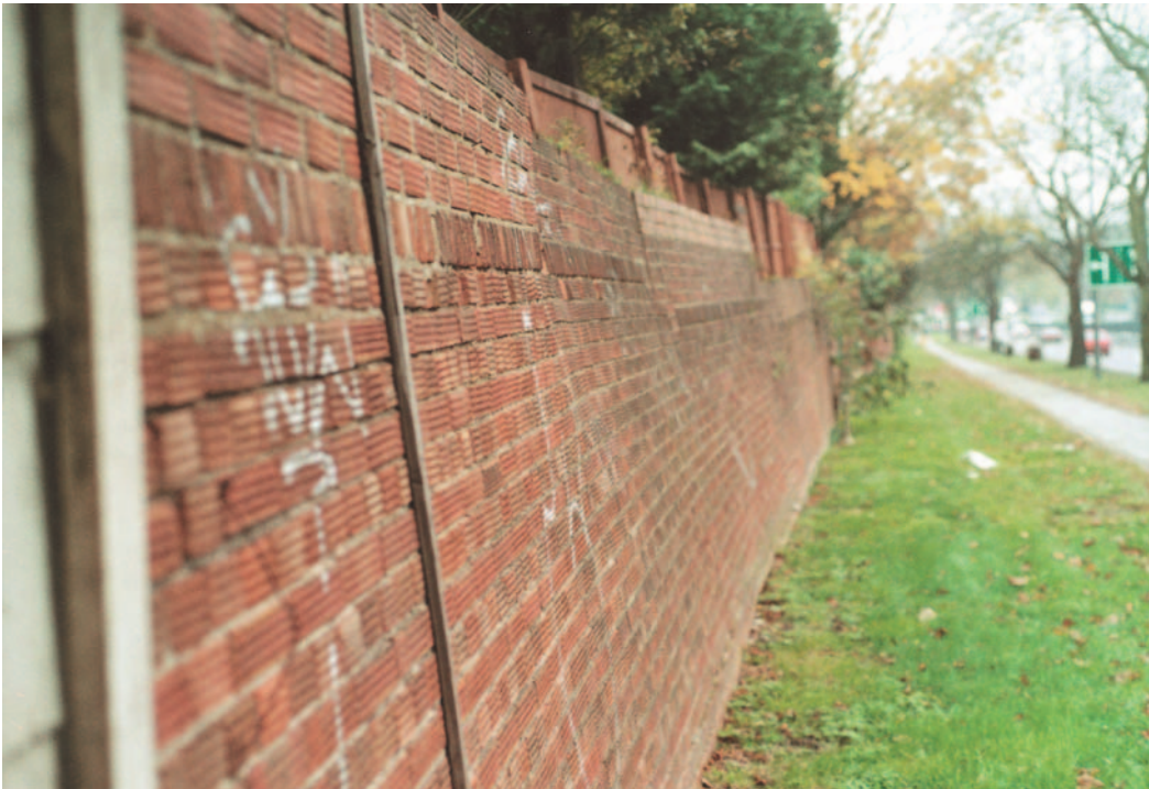
FIG 2.4 If leaning boundary walls have to be rebuilt this can be very expensive.
