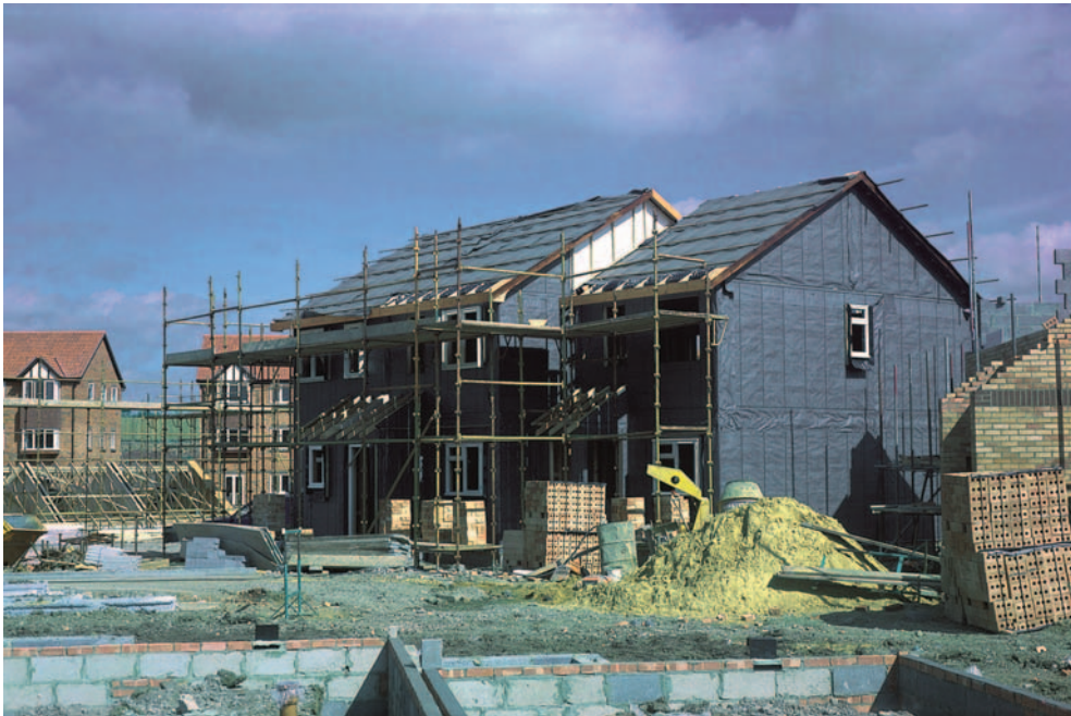
FIG 7.1 Timber frame house under construction in an estate. Note the breather membrane over the timber frame inner skin to the prefabricated timber frame construction.
