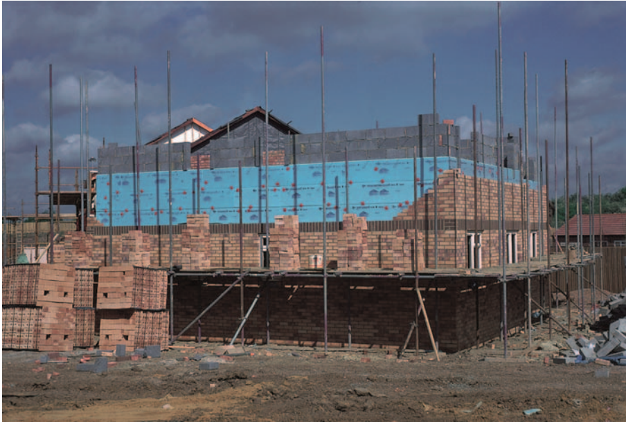
FIG 7.2 A traditional brick and block house under construction in the same estate as the house in Fig. 7.1.
