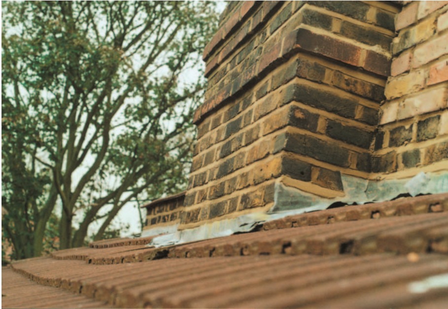
FIG 18.4 Loose and lifting lead flashings will allow driving rain to penetrate.
