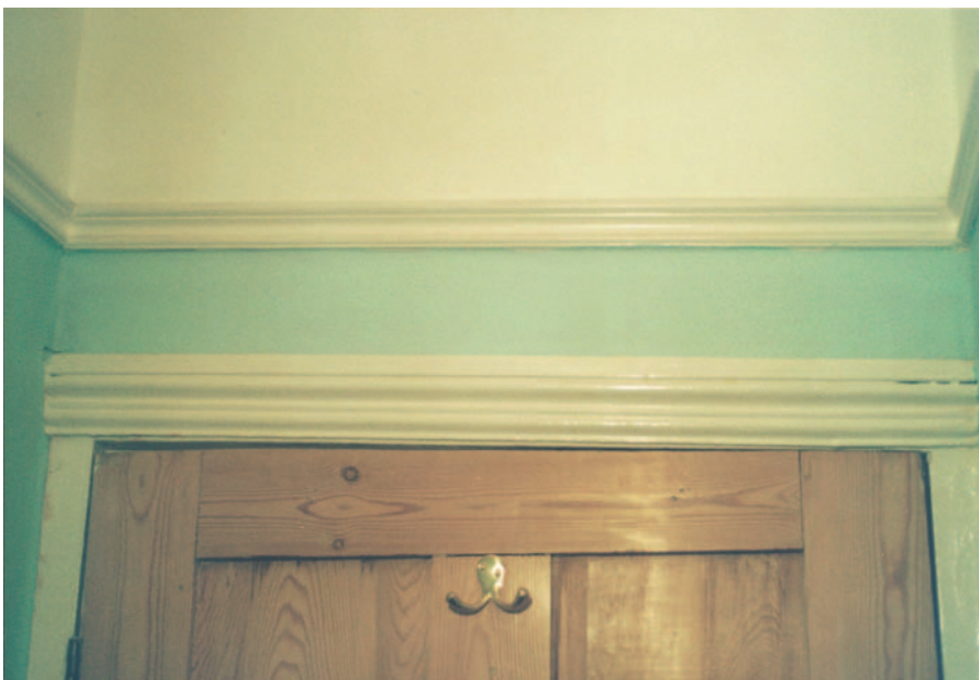
FIG 18.3 Sloping door head due to downward settlement of partition walls.
