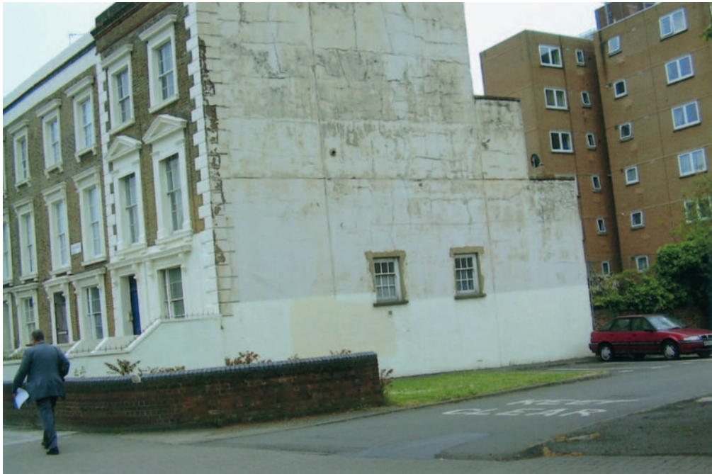
FIG 4.3 Stucco render has been applied to the flank wall of this London terrace. Poor preparation of the wall behind with inadequate keying, trapped moisture and the wrong mix, badly applied, combine to produce this unfortunate result. The builders need to hack it all off back to the brickwork and then start again. Many of these flank walls in London have resulted from Second World War bomb damage, so that part of a terrace has been demolished and something has to be done to weather-proof the exposed wall.
