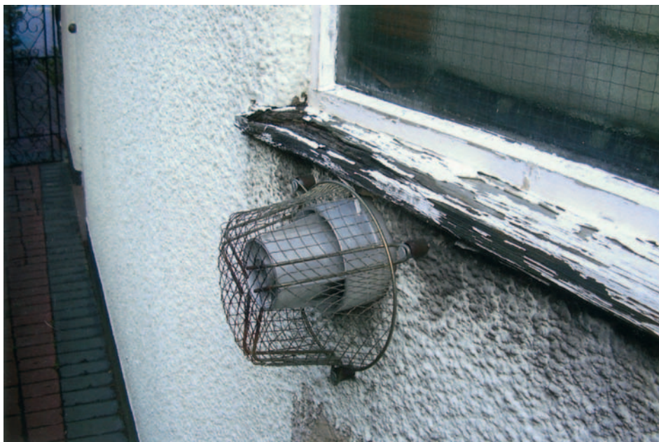
FIG 9.2 The location of this balanced flue directly under the window sill would not comply with current regulations. The discharge of flue gases – mostly water vapour – has had a predictable consequence in the form of wet rot to the window woodwork.
