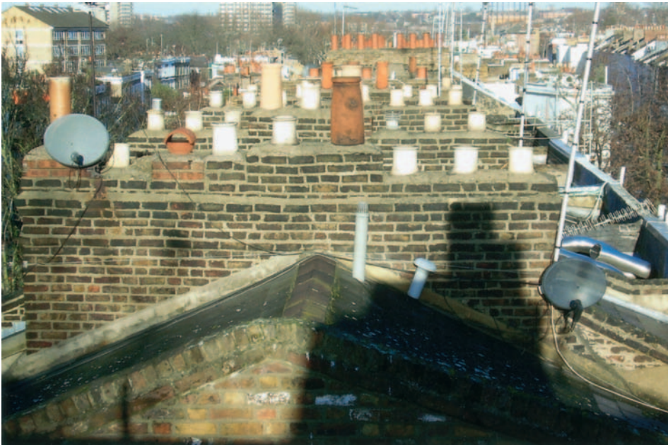
FIG 6.7 In Victorian London almost every room had a fireplace with the flues gathered together in shared chimney stacks over the party walls. Lots of scope here for downward damp penetration. Redundant flues should be vented at the base with hooded pots on top to keep them dry. Often only a limited view will be available from ground level even with the use of binoculars but many of these roofs have external trapdoors from the roofspace, especially the centre-valley or “butterfly” London roofs, so the surveyor can climb out onto the roof to view the construction at close quarters.
