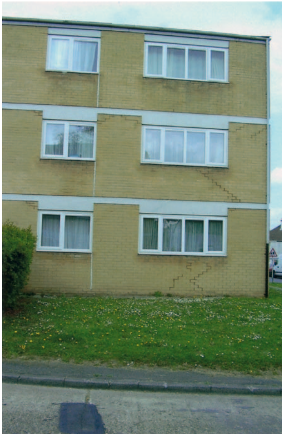
FIG 4.11 These cracks are not related to foundation movements. They are due to differing rates of thermal expansion and contraction between the concrete beamwork and the outer skin to this cavity wall. The cracks have been pointed in a poorly matched mortar, and a vertical sealed movement joint has been added, finished in a white mastic, to accommodate future movement. Potential purchasers may be alarmed by these cracks but in structural terms they are nothing to worry about – they just give the wall a poor appearance. Similar cracking to the plastered blockwork inner skin may present a decorative problem however.
