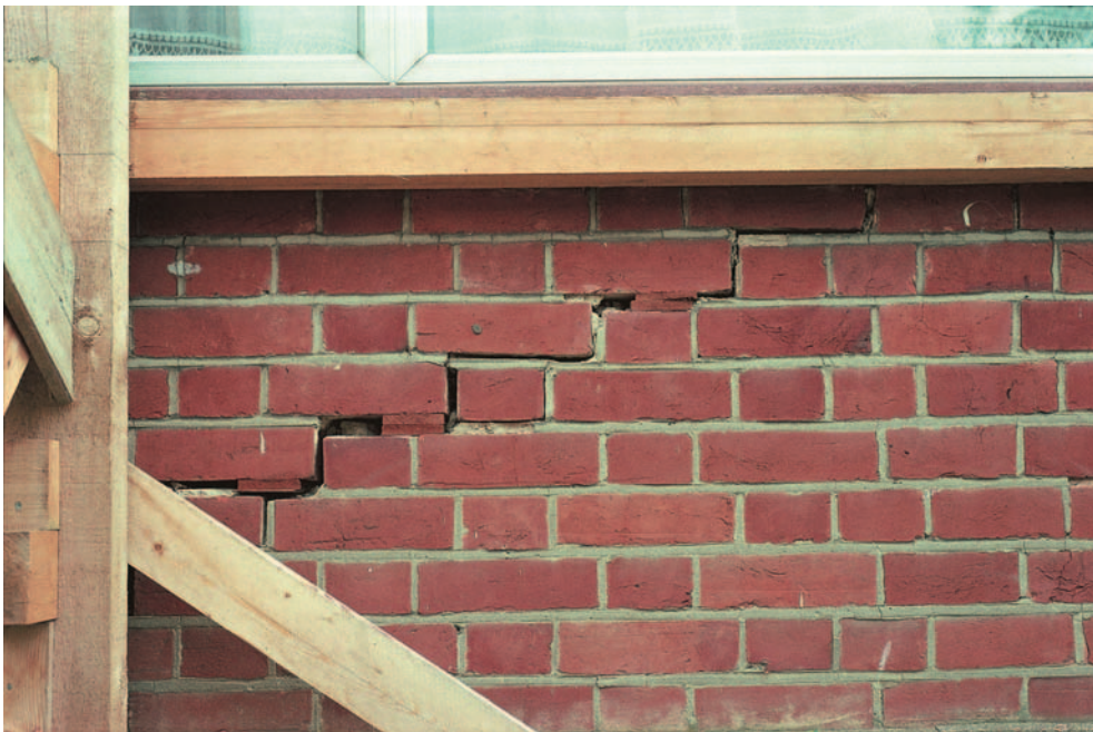
FIG 3.15 Subsidence has affected the lower part of this wall. As a temporary measure raking shores have been placed against the wall and hardwood wedges driven into the open bed joints to prevent further movement of the construction above.
