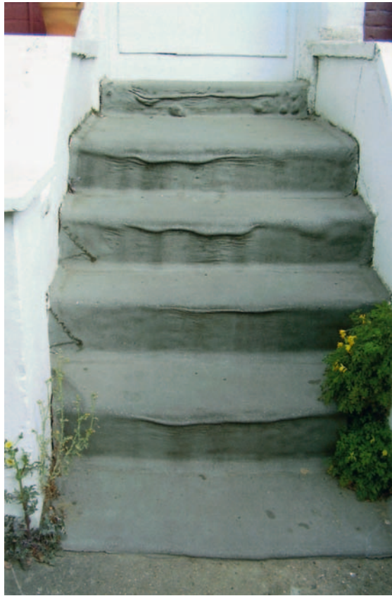
FIG 6.5 Asphalt is used for flat roof covering, basement tanking and as a waterproof surface coating to steps if there are vaults or other accommodation beneath. Vapour blowing and creep can be a problem. Creep to the asphalt on these south-facing steps results from poor preparation and application of the asphalt exacerbated by trapped moisture and exposure to the full heat of the sun.
