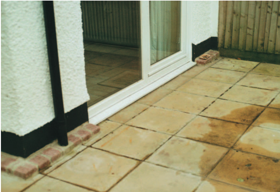
FIG 4.17 The paving is too high. It should be lowered to at least 150 mm (2 brick courses) below the damp-proof course or internal floor level whichever is the lower, with a slope away from the wall.
