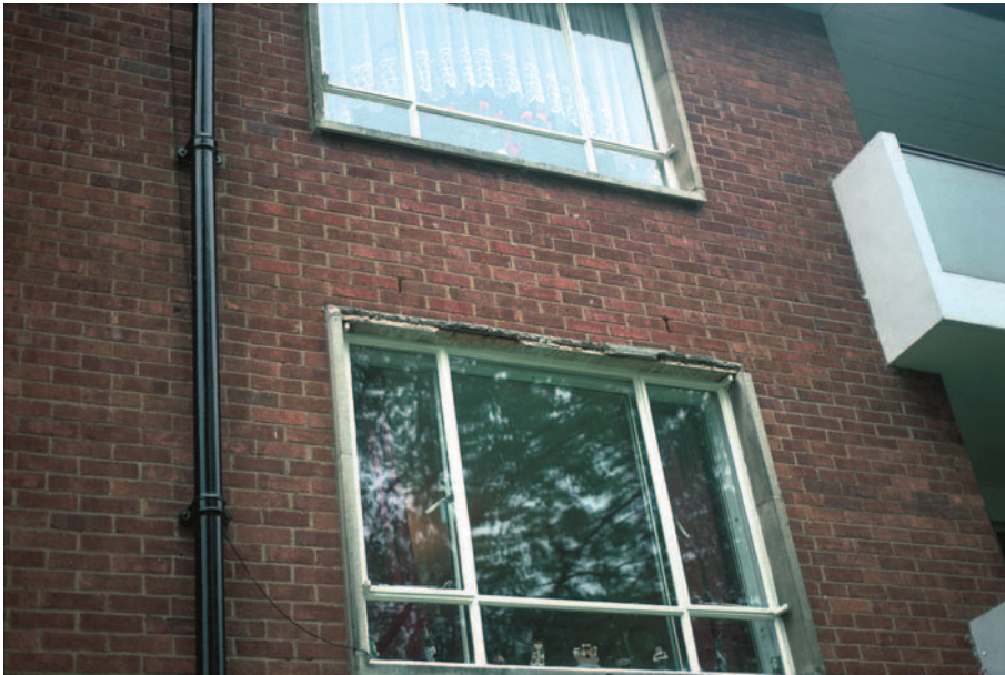
FIG 4.9 Inadequate cover for steel reinforcement in concrete lintel. Rust can take up to seven times the space of the steel it replaces causing bursting to the concrete surface.
