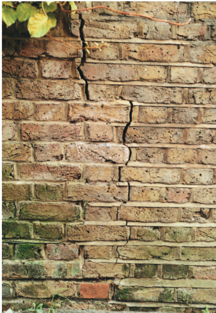
FIG 3.16 Settlement or subsidence again with the crack widening with height.
