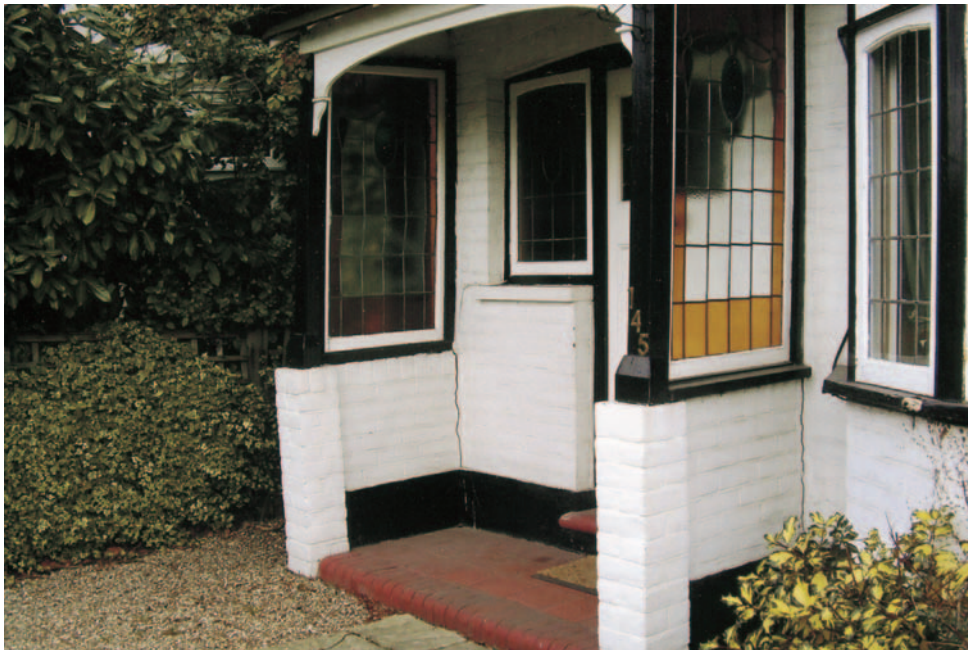
FIG 3.17 Builders will often use a very shallow foundation for a porch thinking that because the weight is low they do not need to excavate as deeply as for the main house; this is not so and the porch in this case will need to be rebuilt on deeper footings.
