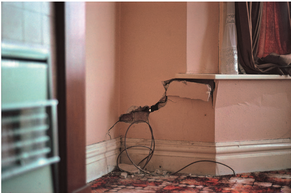
FIG 3.12 Subsidence damage inside house.
