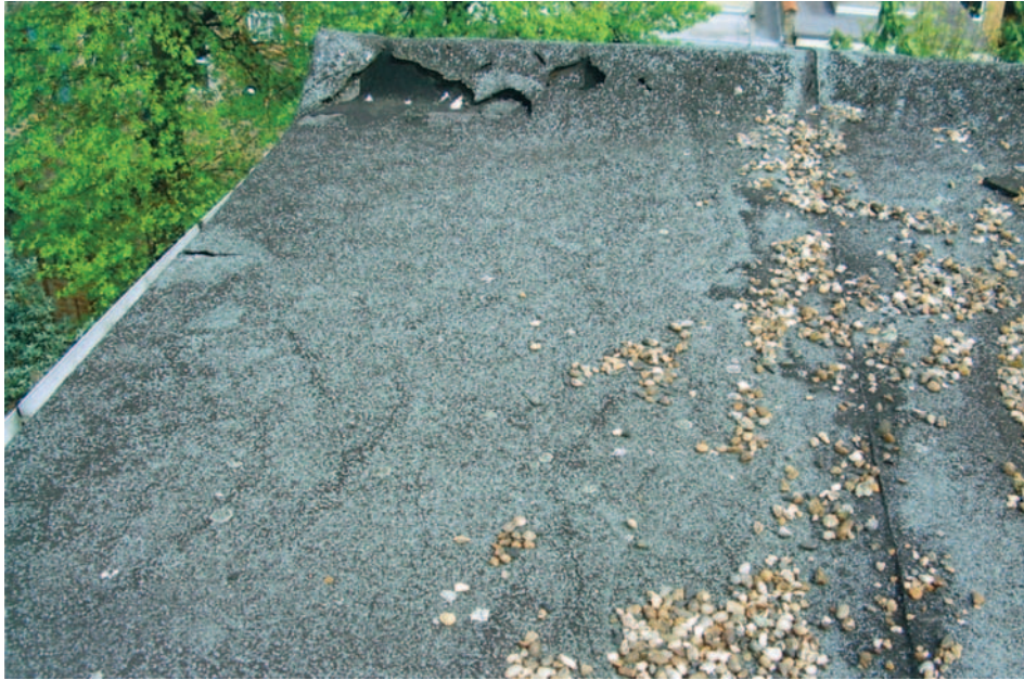
FIG 6.3 A flat roof surfaced in three layers of built-up mineral felt to British Standard 747. Typical life expectancy is less than 10 years. A number of important matters cannot be confirmed without exposure including the condition of timbers, insulation, ventilation under the decking and the presence or otherwise of a vapour barrier. Take care when walking on one of these roofs – the decking may be rotten, and collapse is possible. Watch out for holes cut in the ceiling beneath for downlights, or similar; these can provide a mechanism for warm damp air from the interior to pass into the roof void condensing on timbers and causing premature flat roof failure.
