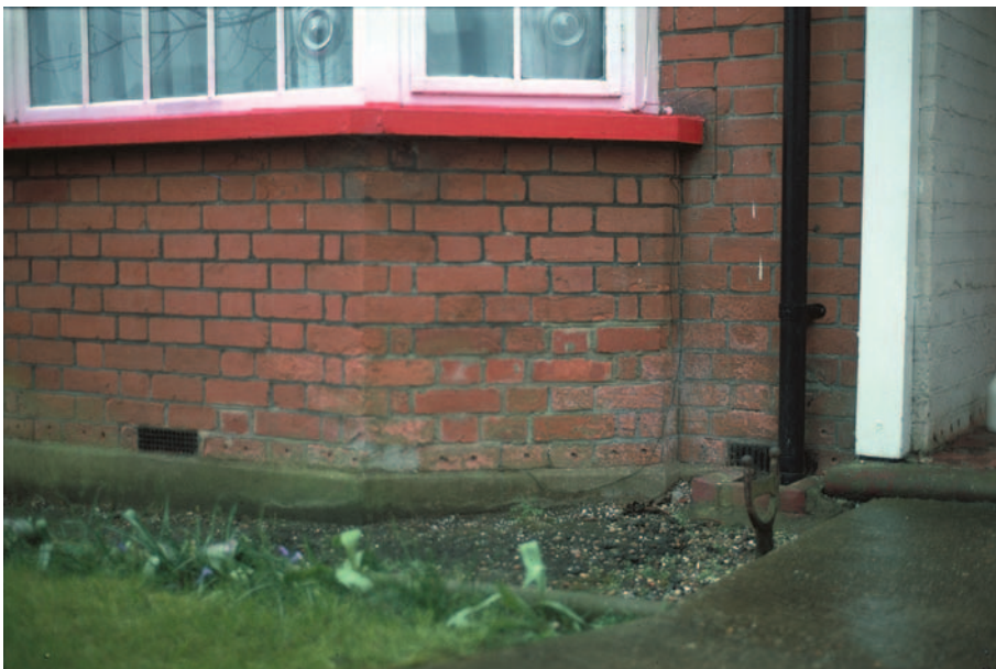
FIG 4.10 Drill holes at the base of the wall indicate that a chemical injection damp-proof course has been added.
