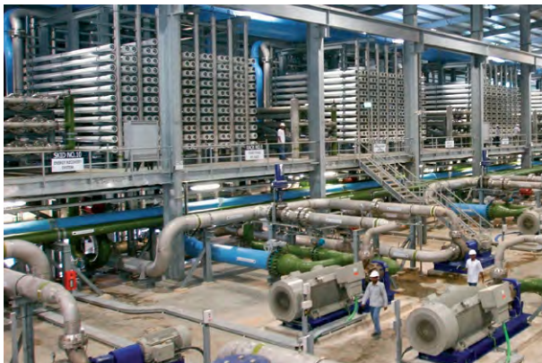
(b) Tuas SWRO plant (136 MI/d), Public Utilities Board, Singapore. (Black & Veatch consultant to EPC contractor, Hydrochem (S) Pte. Ltd.; developer: Hyflux Ltd.; operator: SingSpring Ltd.). (Photo: courtesy of Hyflux).
