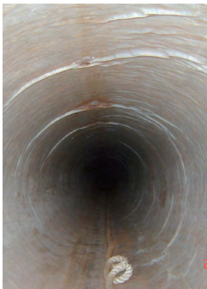
(c) Cure-in-place lining in 600 mm diameter steel pipe. CCTV survey identified defect. (Black & Veatch)
