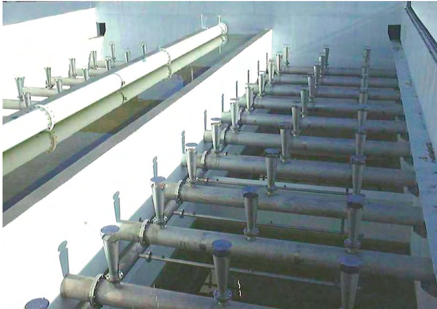
(b) Interior view of a CoCo-DAFF (counter-current dissolved air flotation filtration) clarifier unit.
