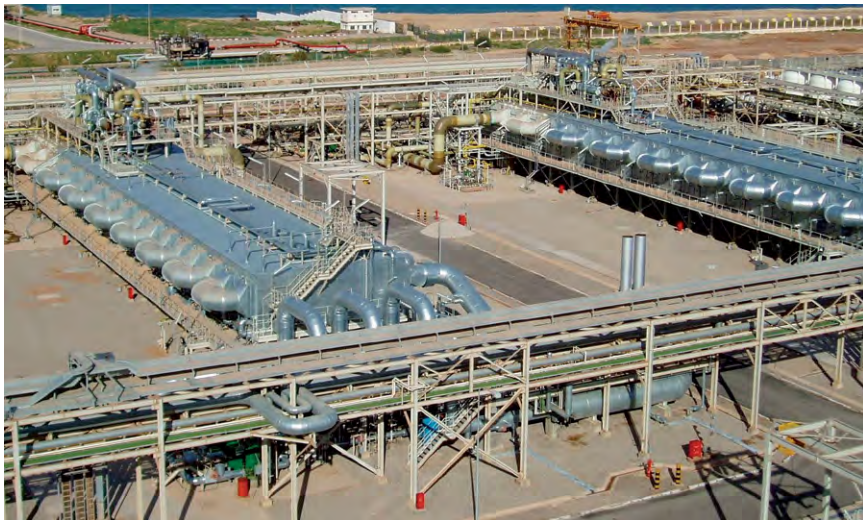
(b) 88 Ml/d multi-stage seawater flash distillation plant with 320 MW output on the Mediterranean coast. (Black & Veatch).
