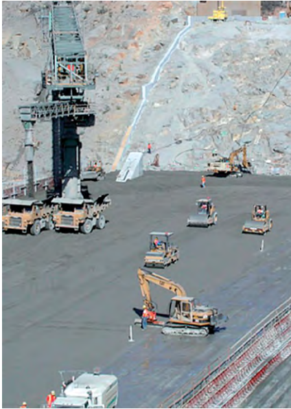
(a) Olivenhain dam under construction, USA. RCC being placed at a rate of about 750 m 3 /hour. (Courtesy of Dr. M. R. H. Dunstan)
