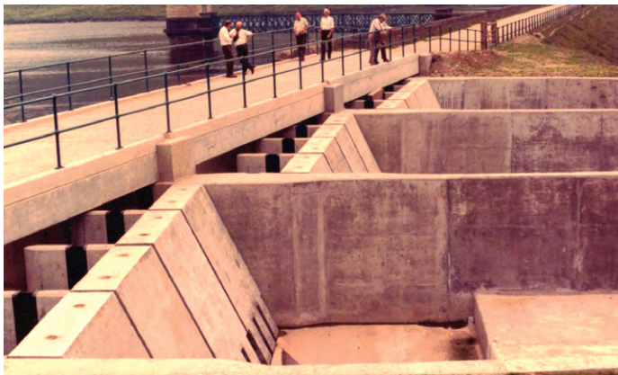
(b) Concrete tipping gates at dam in UK. (Courtesy of John Ackers)
