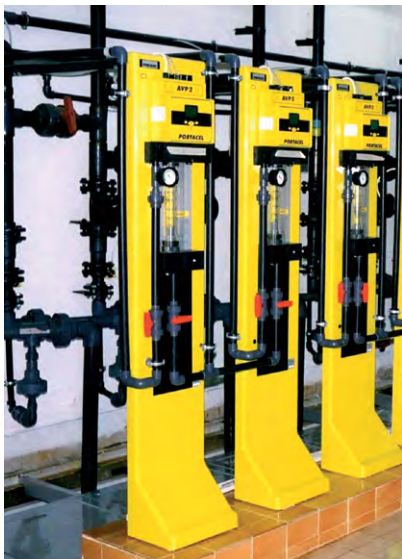
(c) Floor mounted chlorinators. (Manufacturer: Portacel, UK)
