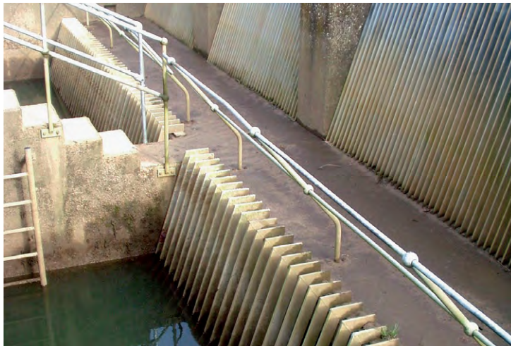
(a) Manually raked bar screens at a river intake in UK.
