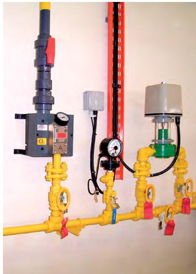
(b) Chlorine gas system with catchpot, changeover device and vacuum regulator. (Manufacturer: Portacel, UK)
