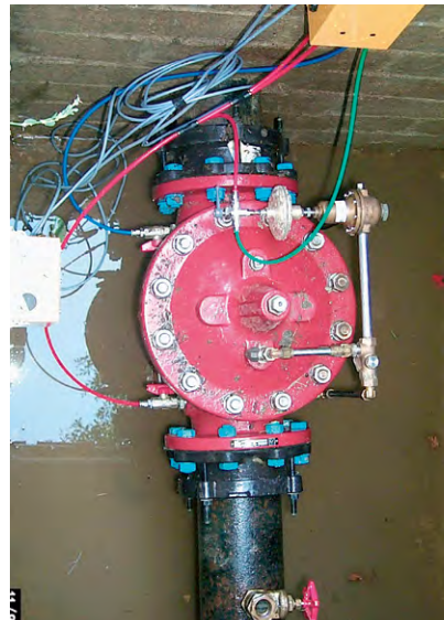
(d) Globe pressure reducing valve in chamber. (Black & Veatch)
