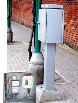
(b) District metering roadside cabinet. Control unit, data logger and pressure gauge. Telemetry and modem can also be installed. (Black & Veatch)
