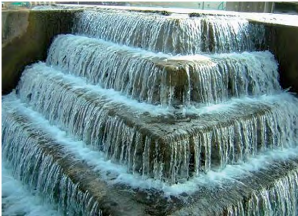
(b) A 4-step cascade aerator (each fall 0.5 m) for 2.75 m 3 /s flow rate at Izmit treatment works, Turkey. (Contractor: Paterson Candy Ltd. UK)
