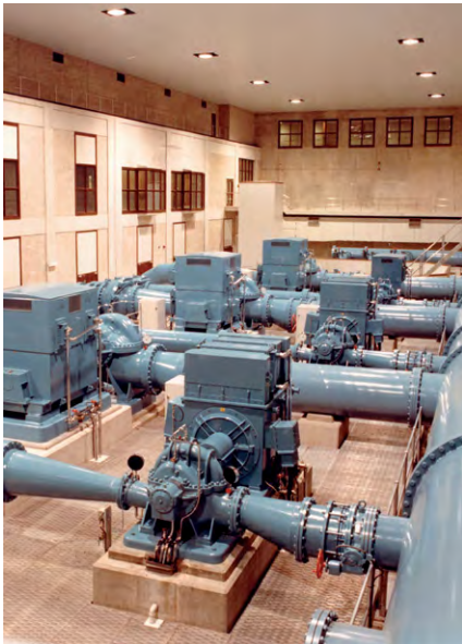
(c) Horizontally mounted double suction centrifugal pumps—1650 m 3 /h @ 53 m lift. (Sulzer Pumps (UK) Ltd.)
