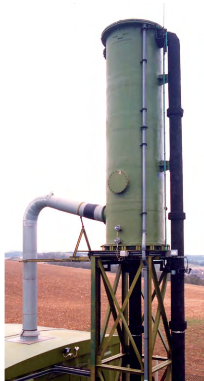
(c) Packed tower aerator of capacity 8 MI/day.
