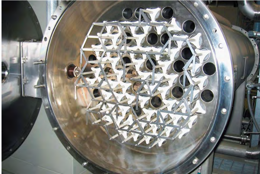
(a) Earl Schmidt Filtration Plant ozone generators, Castaic Lake Water Agency, Santa Clara, CA, USA; capacity 2 \times 17 kg/h @ 10% w/w ozone. (Engineer: Black & Veatch. Manufacturer: Ozonia)
