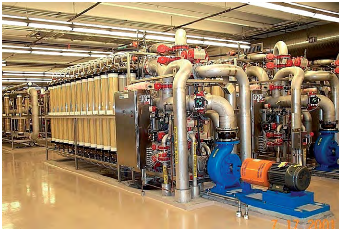
(b) Ultrafiltration membrane system for treatment of lime softened water, capacity 90 000 m 3 /day (Plant location: Mid West USA, System manufacturer: Koch Membrane Systems Inc., Wilmington, MA, USA).
