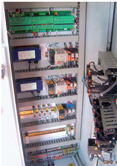
(d) ICA section of MCC with small PLCs and telemetry equipment.
