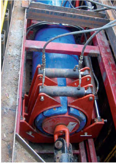
(a) 757 mm OD PE 'swagelining' entering 800 mm diameter host pipe. (Black & Veatch)
