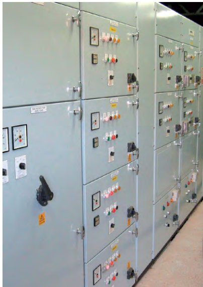
(b) MCC—sections from left to right: incomer and spare; 4 × plant motor starters; cable way; 2 × pump starters; 2 × pump starters.
