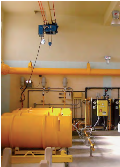
(a) Chlorine drum store with evaporator in the background. (Manufacturer: Portacel, UK; supplier: Bisan Inc. Canada.)
