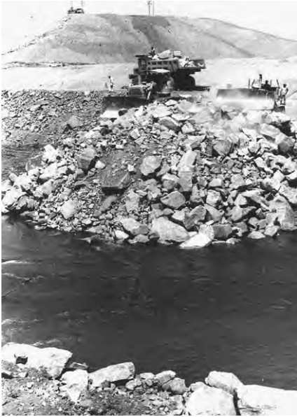
(a) Chira River closure and diversion for Poechos Dam, Peru. (Courtesy of R. L Brown)
