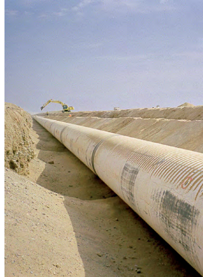
(b) 1524 mm diameter steel pipeline awaiting backfilling in Middle East. (Binnie Black & Veatch)
