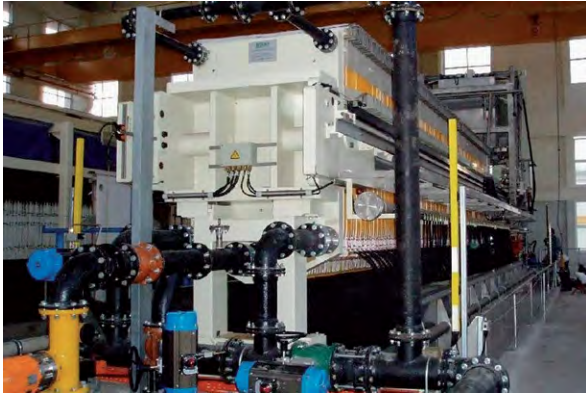
(a) Filter press at the Chestnut Avenue Waterworks, Singapore.
