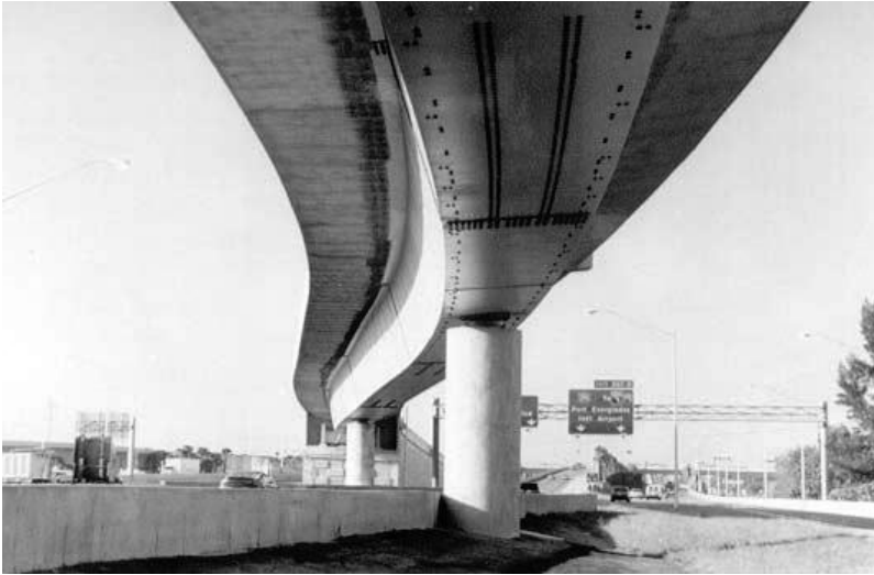
FIGURE 6.5 Single box girder bridge with integral bent cap—Ramp Y, I-95 Davies Blvd, Broward County, FL.
