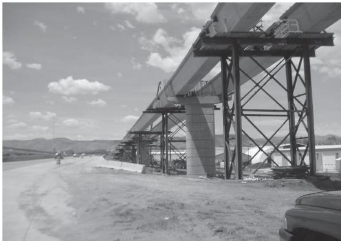
FIGURE 3.32 Precast U girder supported on temporary false-work. (Courtesy of Summit Engineering Group.)
