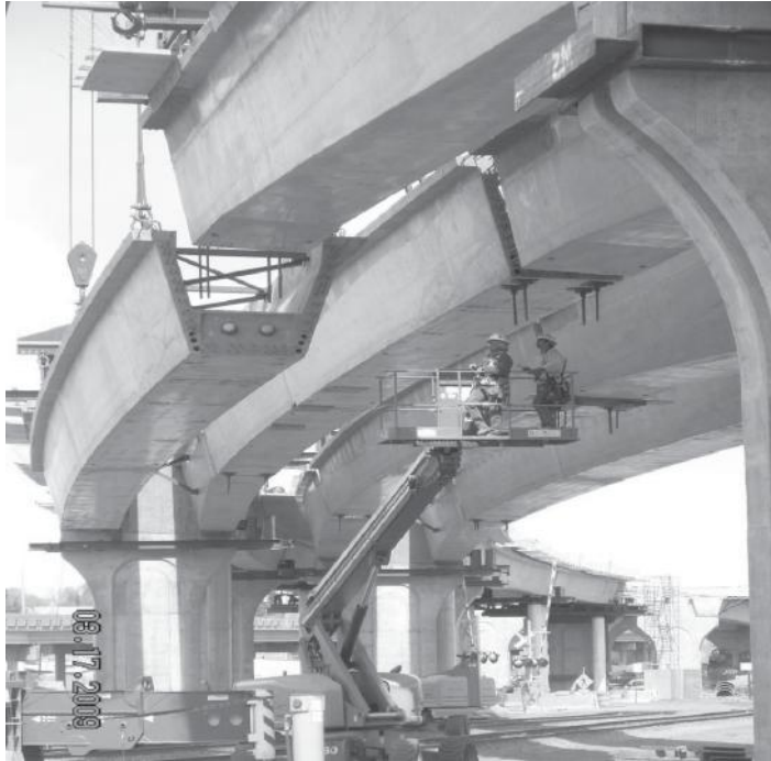
FIGURE 3.31 Precast spliced U girder bridge during erection. (Courtesy of Summit Engineering Group.)
