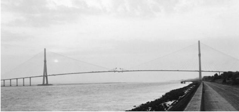
FIGURE 10.24 Normandy Bridge, France, completed in 1995. Main span 856 m. The photo shows the final stage of construction just prior to main span closure. (Courtesy of COWI A/S [S. Lausten].)
