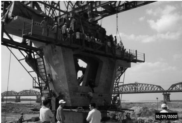
FIGURE 3.18 Split precast pier segment.
