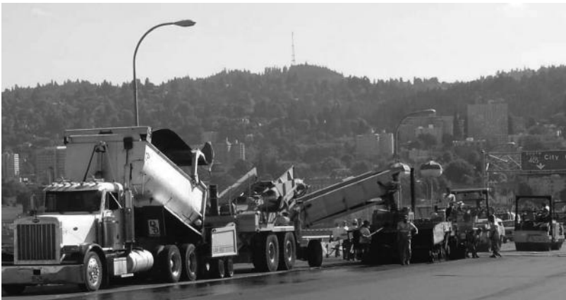
FIGURE 16.45 Paving train of equipment for constructing a wearing surface. (Courtesy of Charles Seim.)
