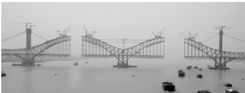
FIGURE 8.43 Free cantilever method used in the Dashengguan Bridge in China. (Courtesy of Kangming Chen.)
