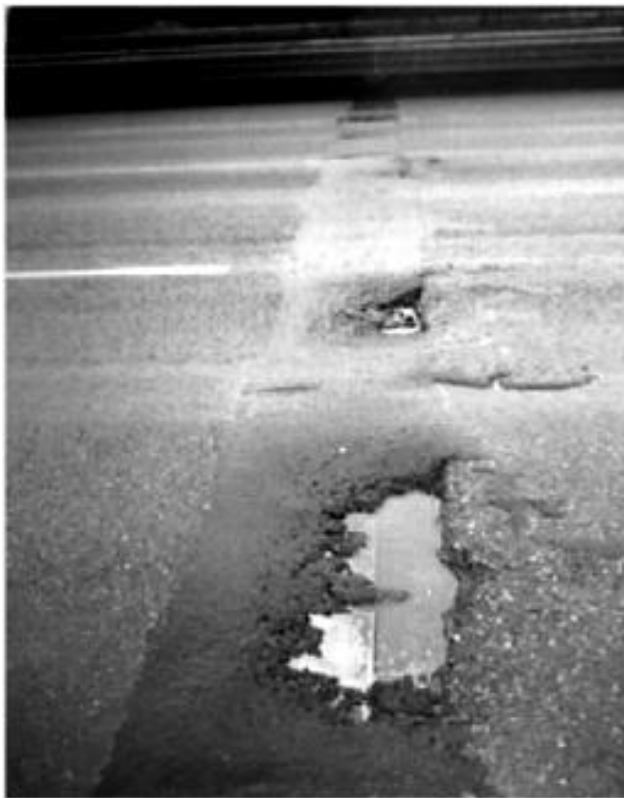
FIGURE 18.7 Failed asphaltic plug joint application.
