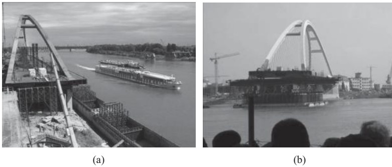
FIGURE 8.53 Apollo Bridge, Slovakia ( http://www.most.pokorny.sk/ ): (a) assembly at river bank and (b) floating of arch span to its final position.
