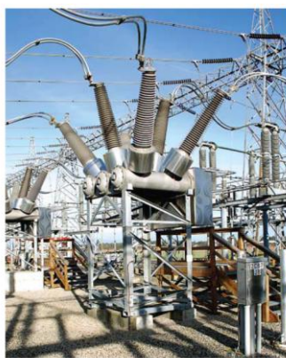
230 kV SF_6 Dead Tank
