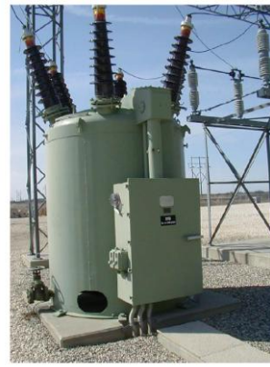
69 kV Oil Dead Tank
