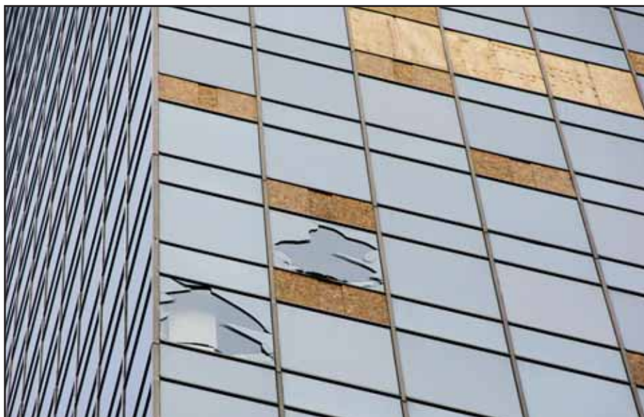
Glazing damage due to roof aggregate from adjacent building in Hurricane Ike
