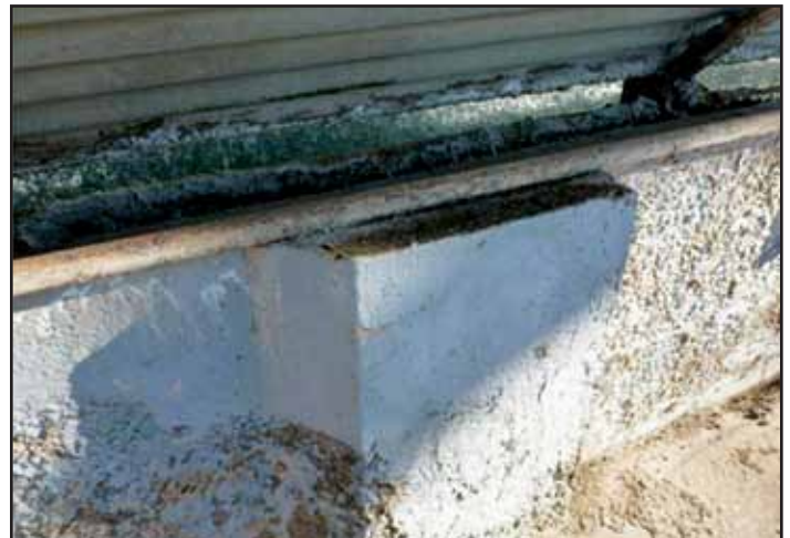
Figure No. 5 View of eroded exterior concrete Basin Wall surfaces adjacent to the Chemical-Charging Station.
