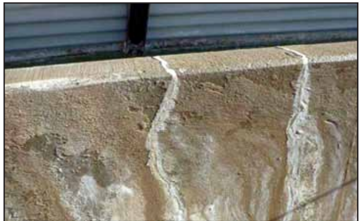
Figure No. 9 View of failed crack sealant repairs on exterior Basin Walls.
