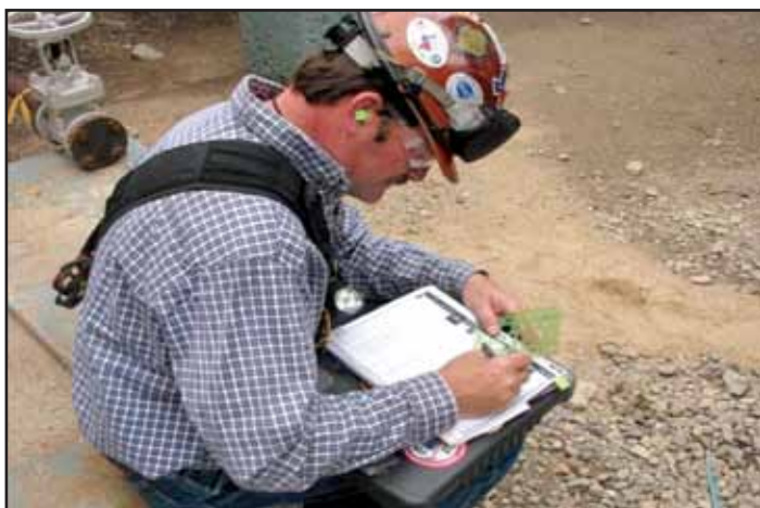
Figure No. 1 Deterioration mapping of observed exterior structural concrete members
