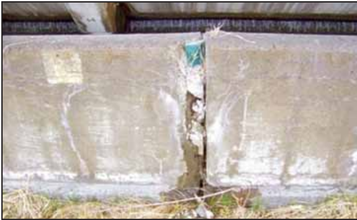
Figure No. 6 Failed Expansion Joint.
