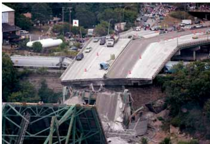
Figure 1: Photo of Minnesota bridge collapse [2]
