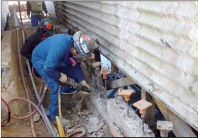
Figure No. 10 Extensive Basin Wall section-losses due to freeze-thaw damage and aggressive chemical attack.
