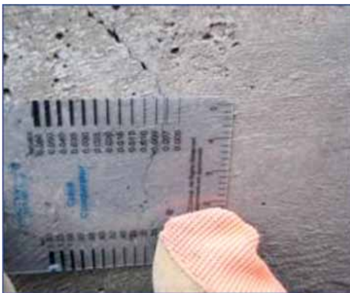
Figure No. 4 Crack Comparator measurement of crack widths
