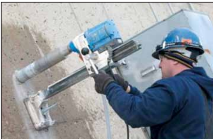
Figure No. 8 Concrete core sampling of a Natural Draft Hyperbolic Cooling Tower Veil.
