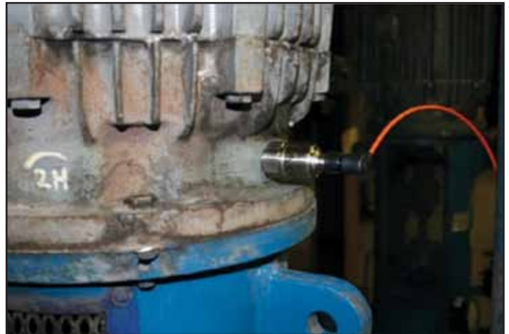
Figure 9: Permanently mounted accelerometer on a motor.
