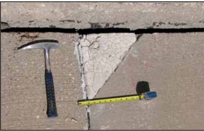
Figure No. 7 View of failed precast concrete repairs on exterior Canopy Panels.
