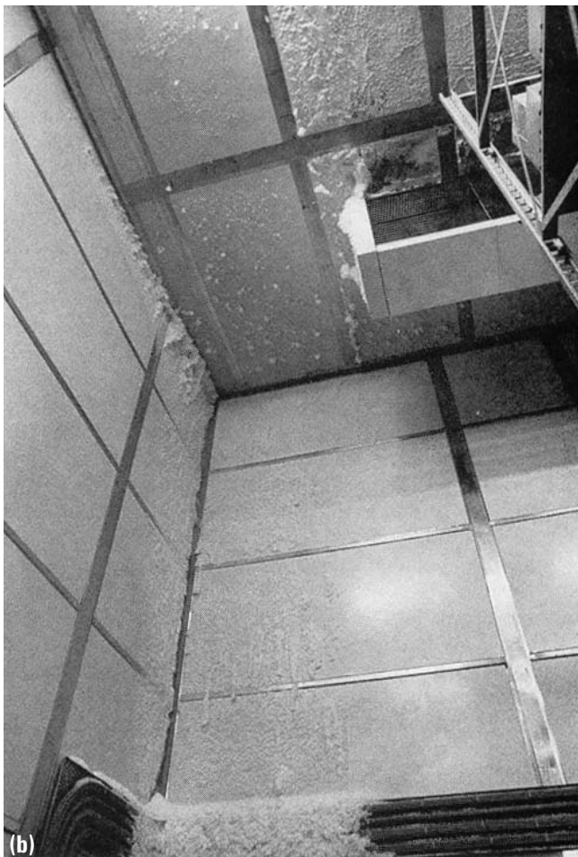
Figure 6.19 (a) Plastic faced plywood cladding spalled off by ice build-up. Ice accumulation can be seen on the output face. (b) Output side of cooler bank is badly positioned, near a corner and frequently opening door. Ice is spread into the corner by the fans, and down to cover electric trunking.
