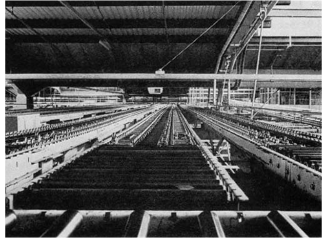
Figure 4.175 Combinations of powered and free conveyors in factory.
