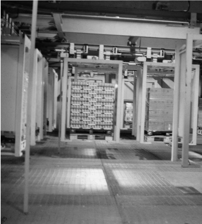
Figure 4.193 Monorail conveyor used between automated warehouse and order picking area: each carrier is individually powered and can run at 1.8 m per second.
