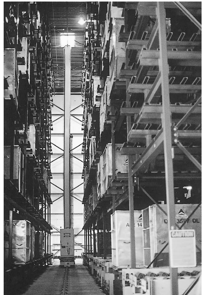
Figure 5.17 Stacker crane – note structural racking with air cargo containers resting on 'top hat' sections.
