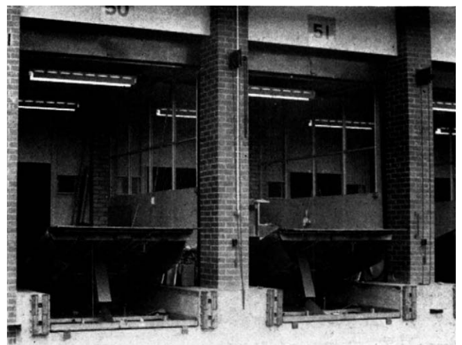
Figure 2.56 Hydraulic dock leveller. These are for light vans and so are nearer the ground than usual.
