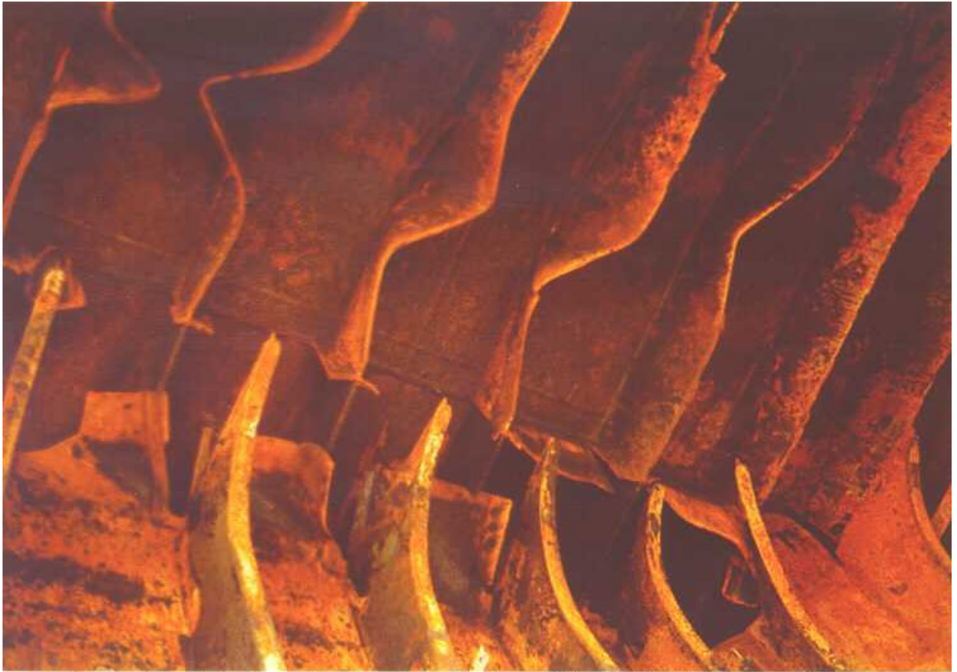
No. 17 — shows the buckling of the deck longitudinals in the port PBT and the forward displacement of transverse bulkhead 79. It will be noted that the deck longitudinals in the No. 3 wing tank are not buckled.
